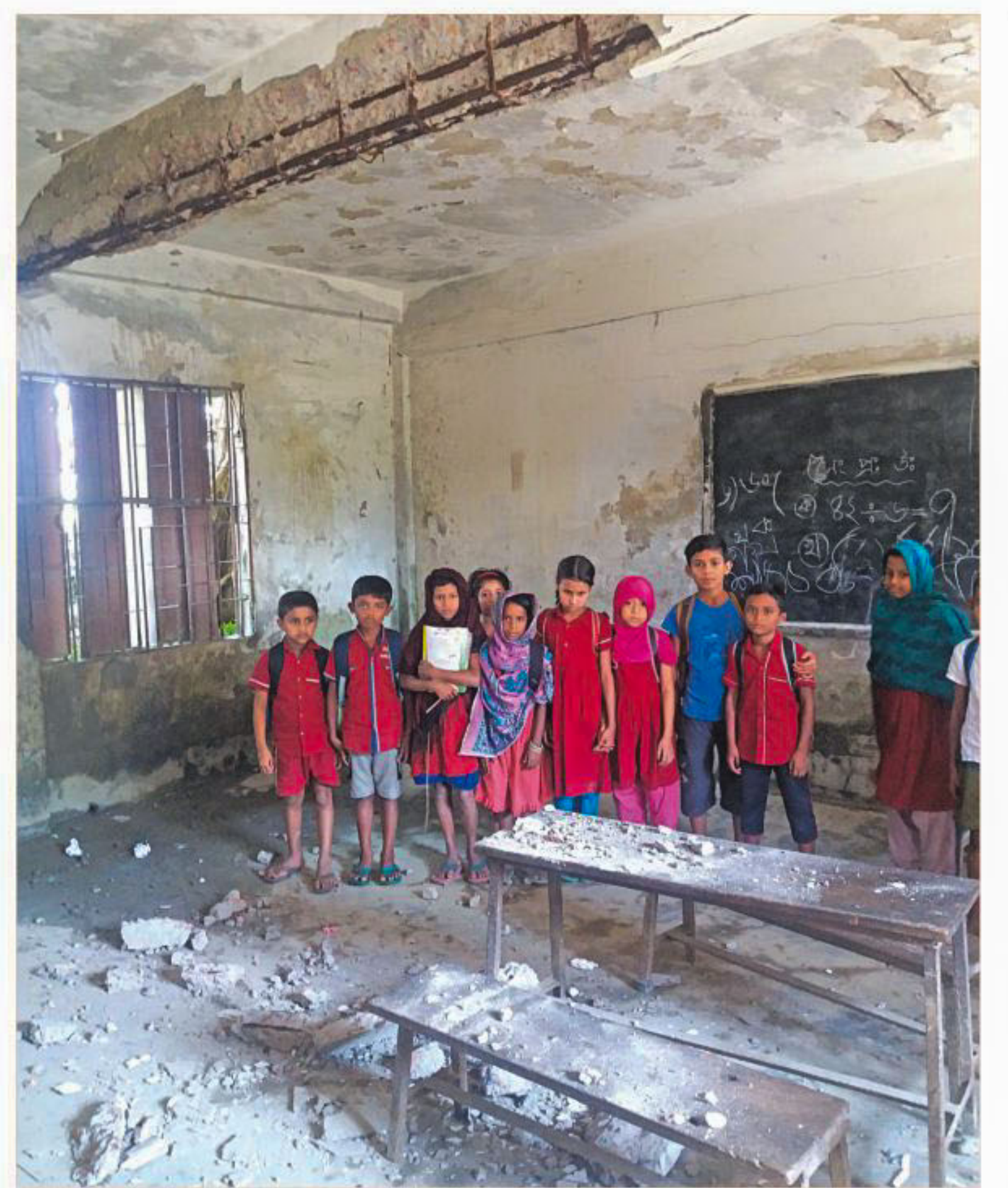
Schoolchildren look at the debris in their classroom at Chandukhali Govt Primary School in Patuakhali's sadar upazila. A number of students were hurt after parts of the worn-out roof collapsed on them during their class yesterday.
