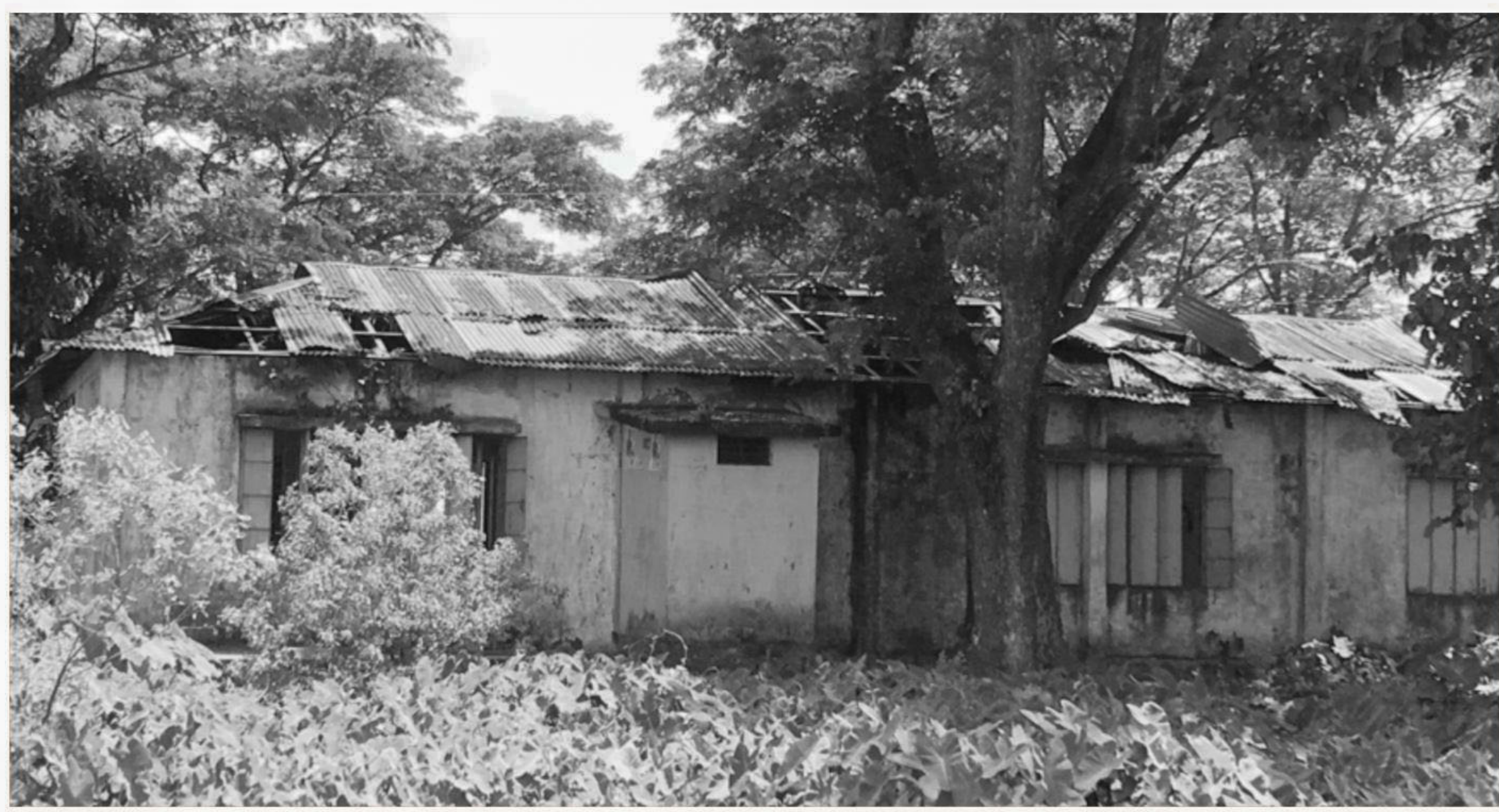
Like several others of the kind, the building of Sarompur Government Primary School in Rajnagar upazila under Moulvibazar district remains in an awfully dilapidated condition, posing risk for students and teachers.
