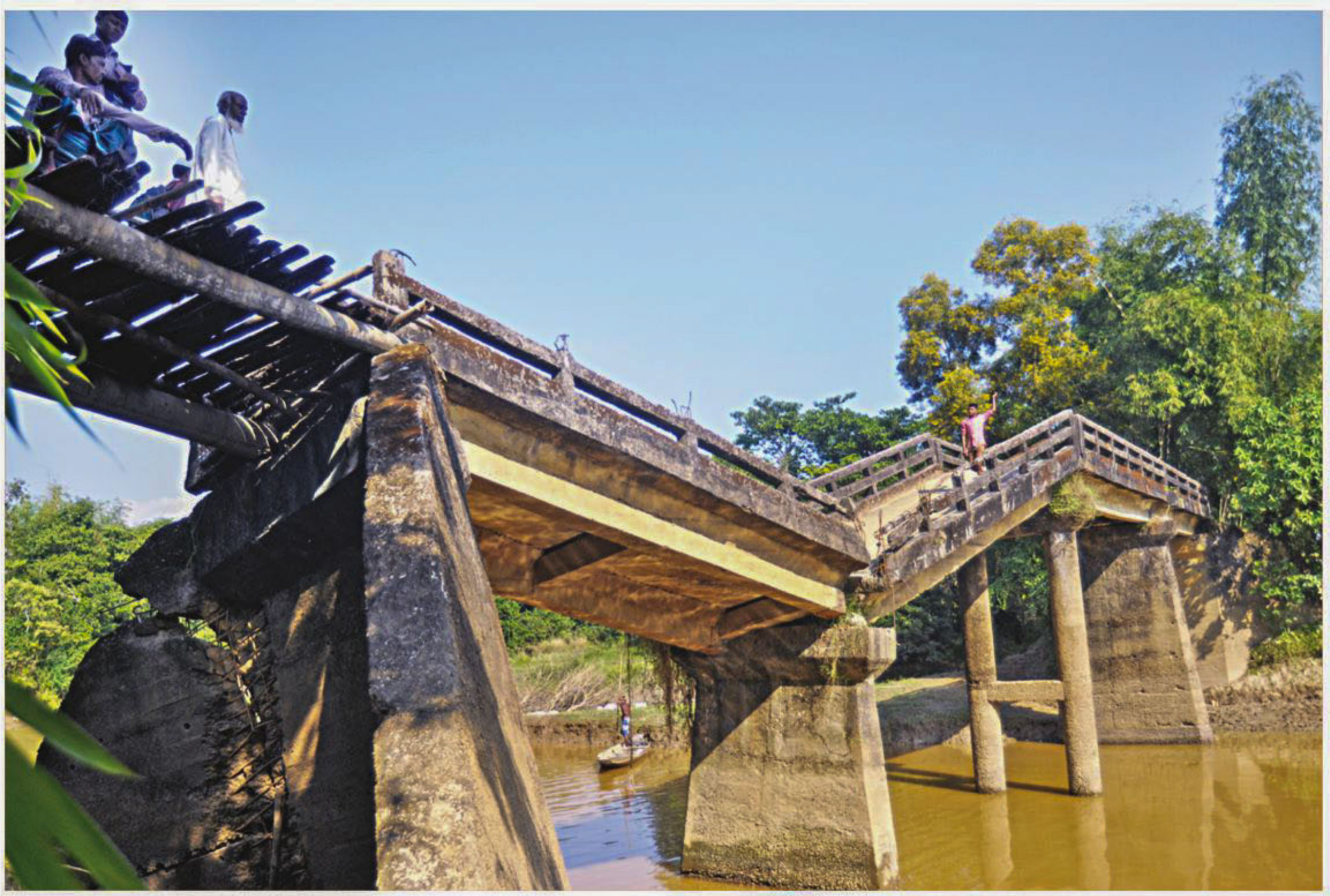
It is hard to believe but Shikor Khai Bridge at Bilaimara village of Jaintapur upazila in Sylhet has been lying like this for decades after partially collapsing some 33 years back. Governments come and go, but none bothers to take care of the bridge around 25,000 people including schoolchildren of 15 villages use, putting their lives at grave risk. The photo was taken on Monday.
