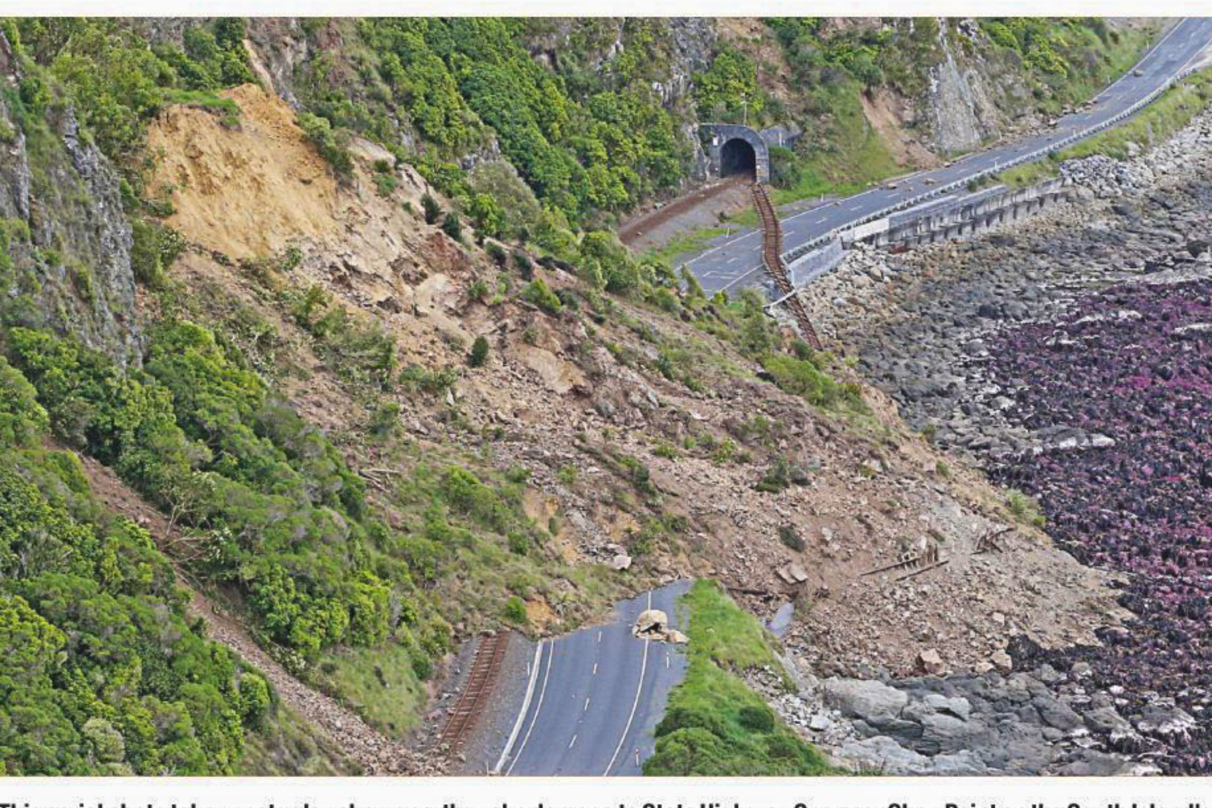
This aerial photo taken yesterday shows earthquake damage to State Highway One near Ohau Point on the South Island's east coast, New Zealand. Top right, a woman and child in front of a house damaged by the earthquake. Bottom right, locals look at damage caused by the earthquake along State Highway One near the town of Ward on South Island yesterday.
