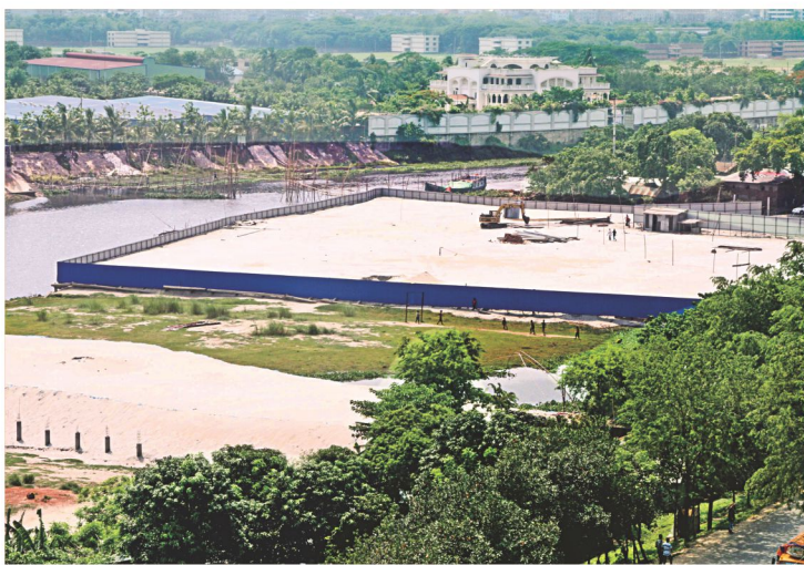
The photo taken in May shows earth filling going on inside a fence built occupying a portion of the Turag near Kamarpara Bridge in Tongi. The High Court yesterday directed the government to stop earth filling, encroachment and construction of structures along the Turag in 48 hours.
