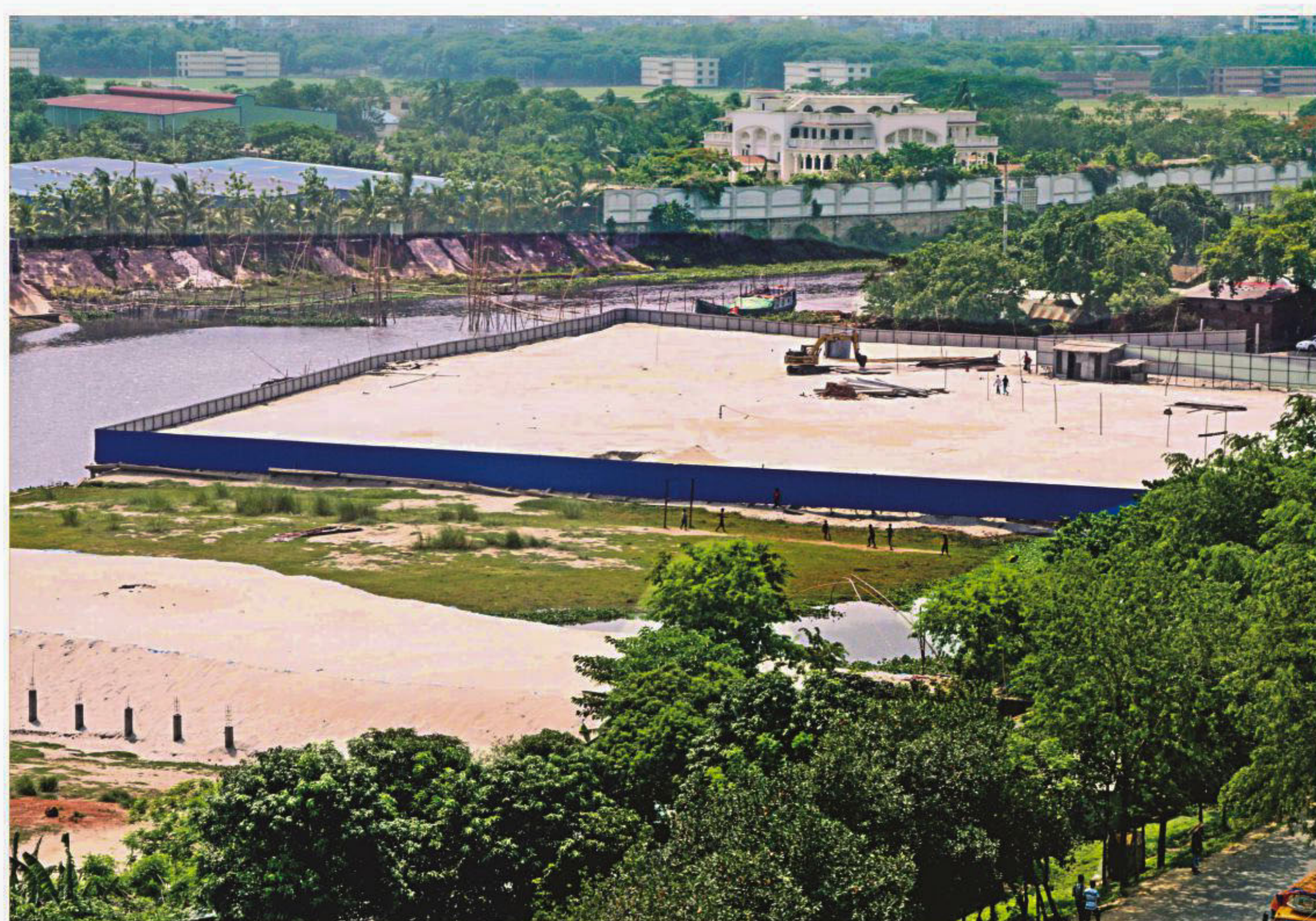
The photo taken in May shows earth filling going on inside a fence built occupying a portion of the Turag near Kamarpara Bridge in Tongi. The High Court yesterday directed the government to stop earth filling, encroachment and construction of structures along the Turag in 48 hours.
