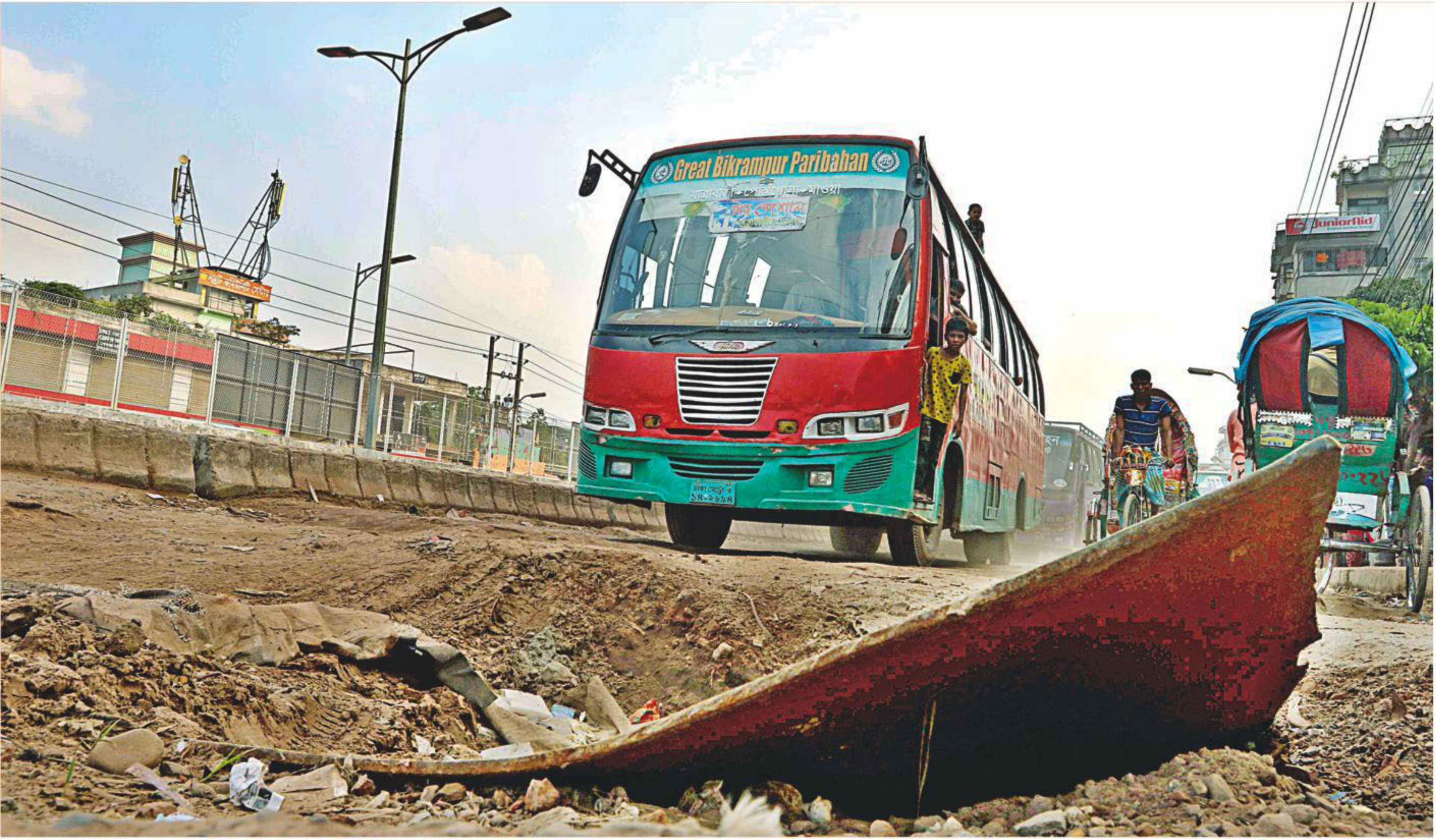
A damaged steel plate over a sewerage drain on the road under Mayor Mohammad Hanif Flyover near the capital's south Jatrabari has been left like this for a while, posing risk of accidents. The road is also plagued with potholes, making it difficult to access, mainly due to poor maintenance and repair by the city corporation. The photo was taken yesterday.
