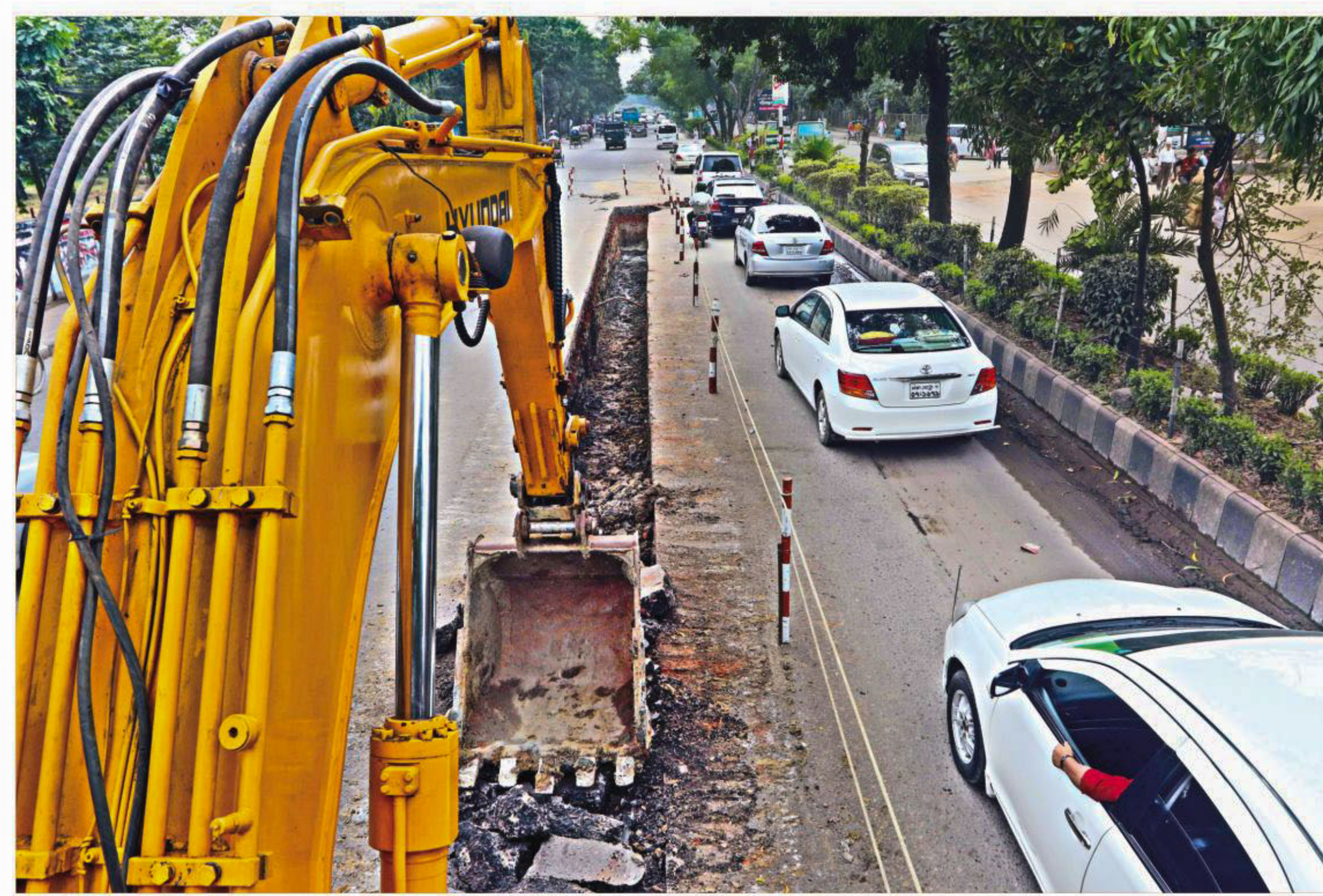
An excavator digs a trench on Begum Rokeya Sarani near IDB Bhaban in the city to relocate an underground 132kv power cable yesterday. The work is part of the metro rail construction project. PHOTO: PRABIR DAS
