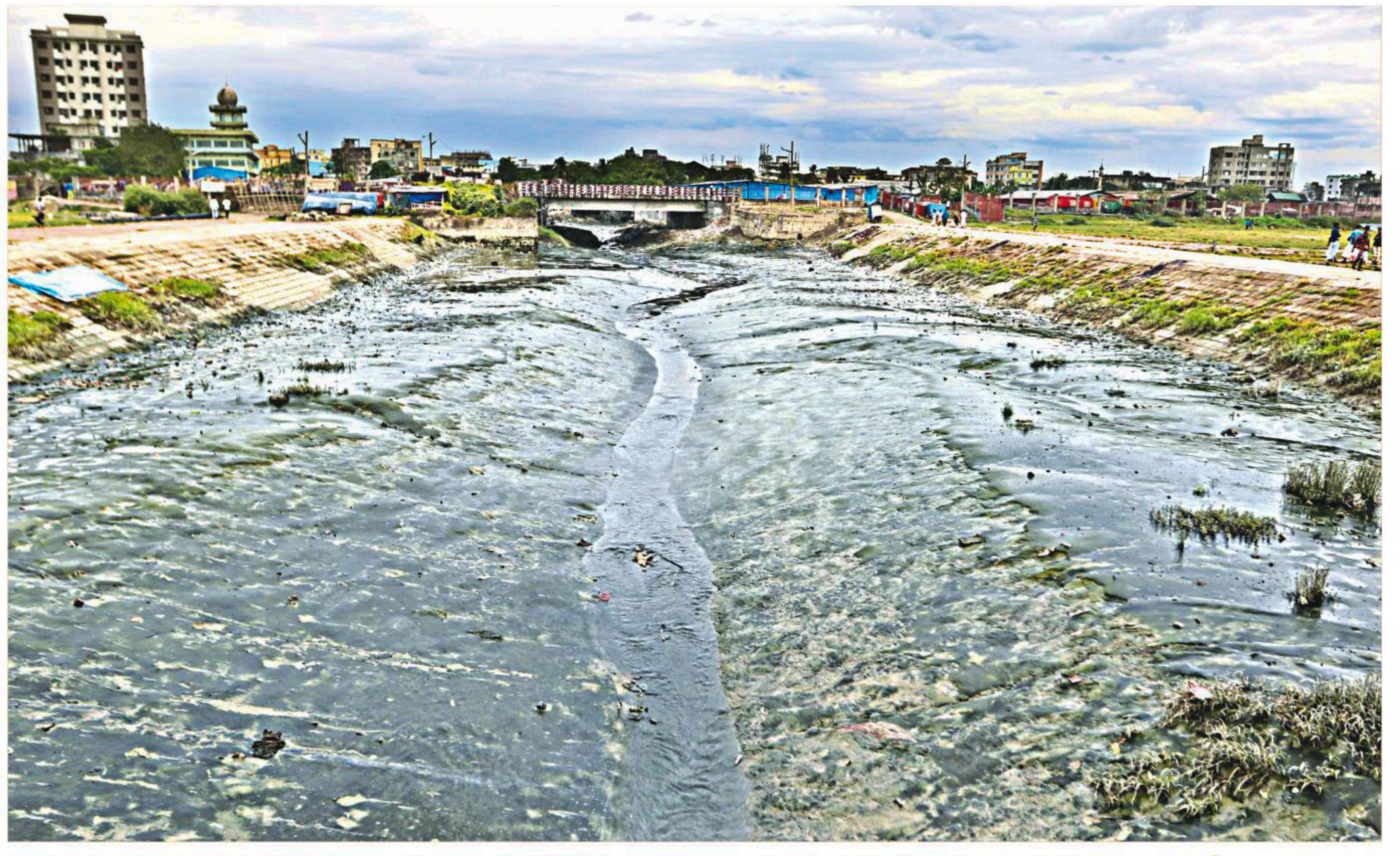
The flow of water is about to be blocked in Firingi Bazar canal, which drains rainwater to the Karnaphuli river from different areas of Chittagong city, with the water body being silted. The photo was taken in the port city's Firingi Bazar area yesterday.
