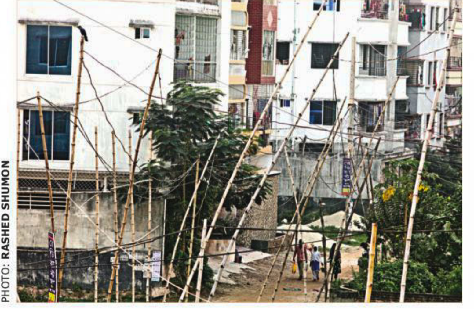
People walk underneath a cobweb of electric lines held up by slanting bamboo poles posing risk of fatal accidents. The photo was taken recently in the capital's south Banasree area.
