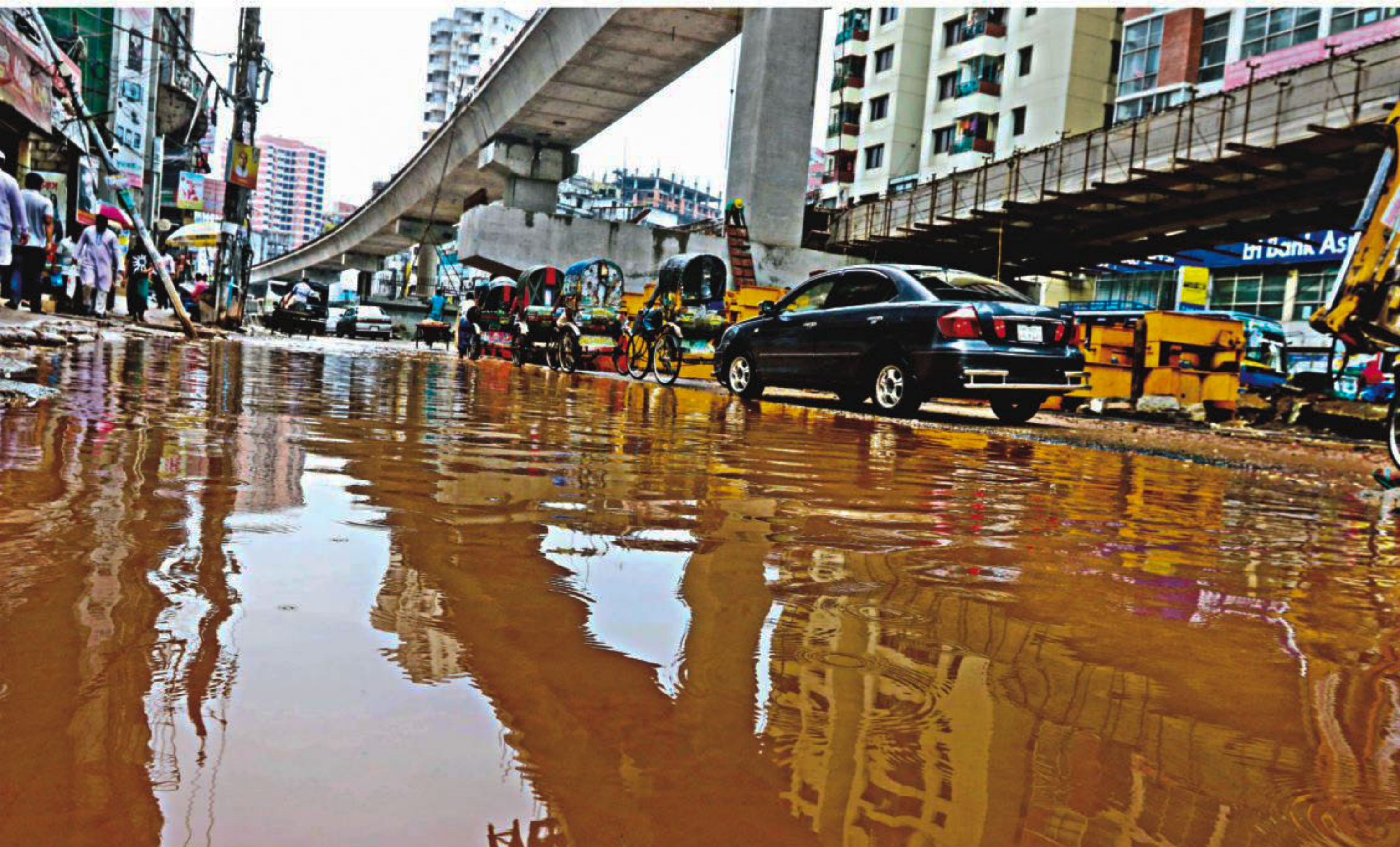
Travelling along this road from Malibagh to Shantinagar in the capital has turned into a nightmare as one has to cross numerous muddy water-filled potholes. The photo was taken yesterday.
