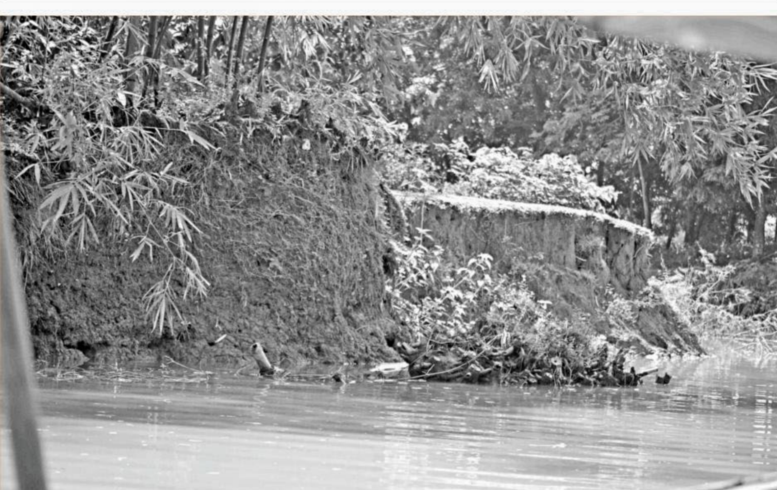
A section of the bank of the Moheshkhola river in Isamari village under Dharmapasha upazila of Sunamganj is in danger of being washed away by the river. Five other villages of the upazila face the same risk.
