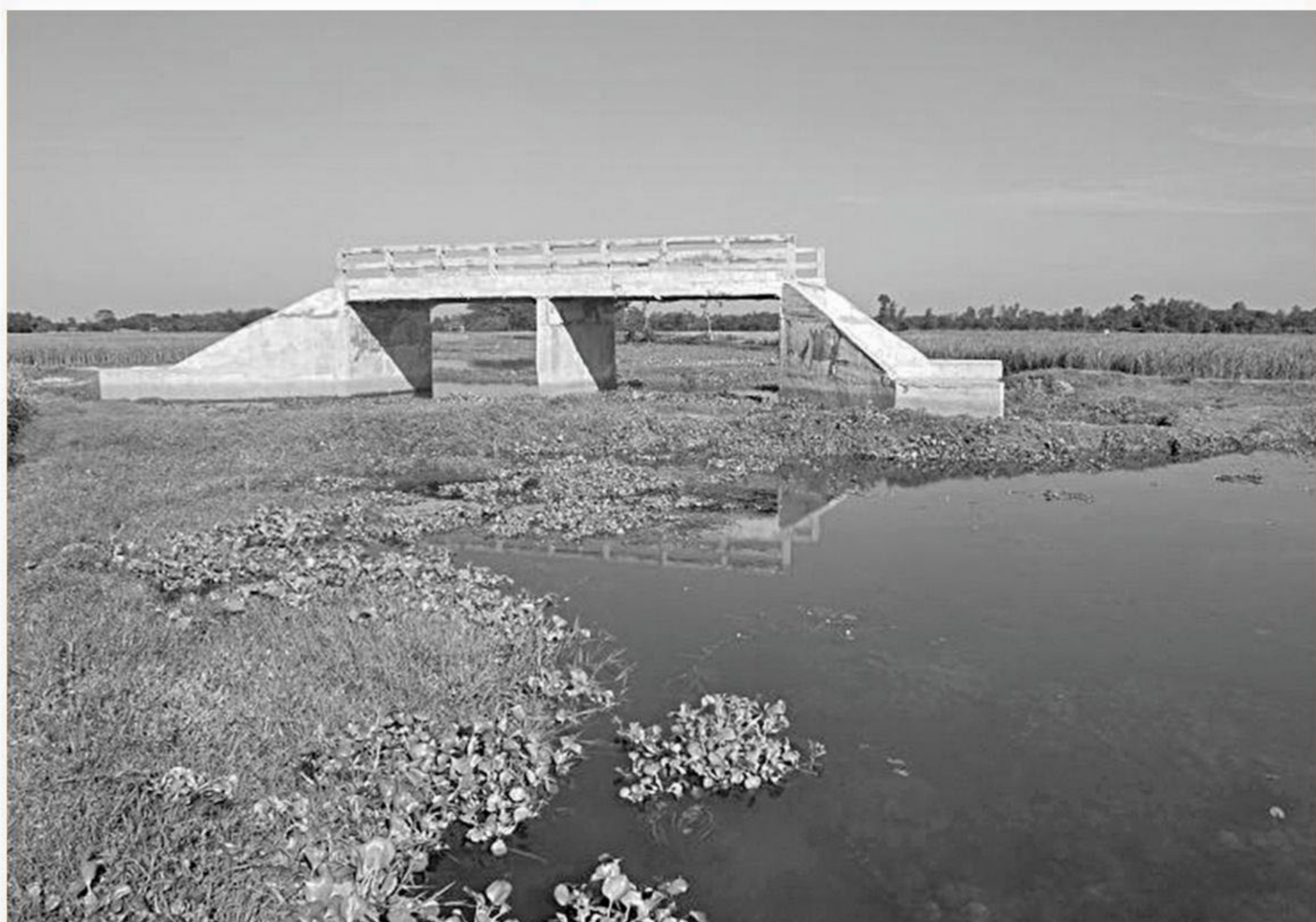
This concrete bridge over a canal at Ismailer Dola village in Kishoreganj upazila of Nilphamari remains useless since completion of its construction about six months ago due to lack of approach roads.
