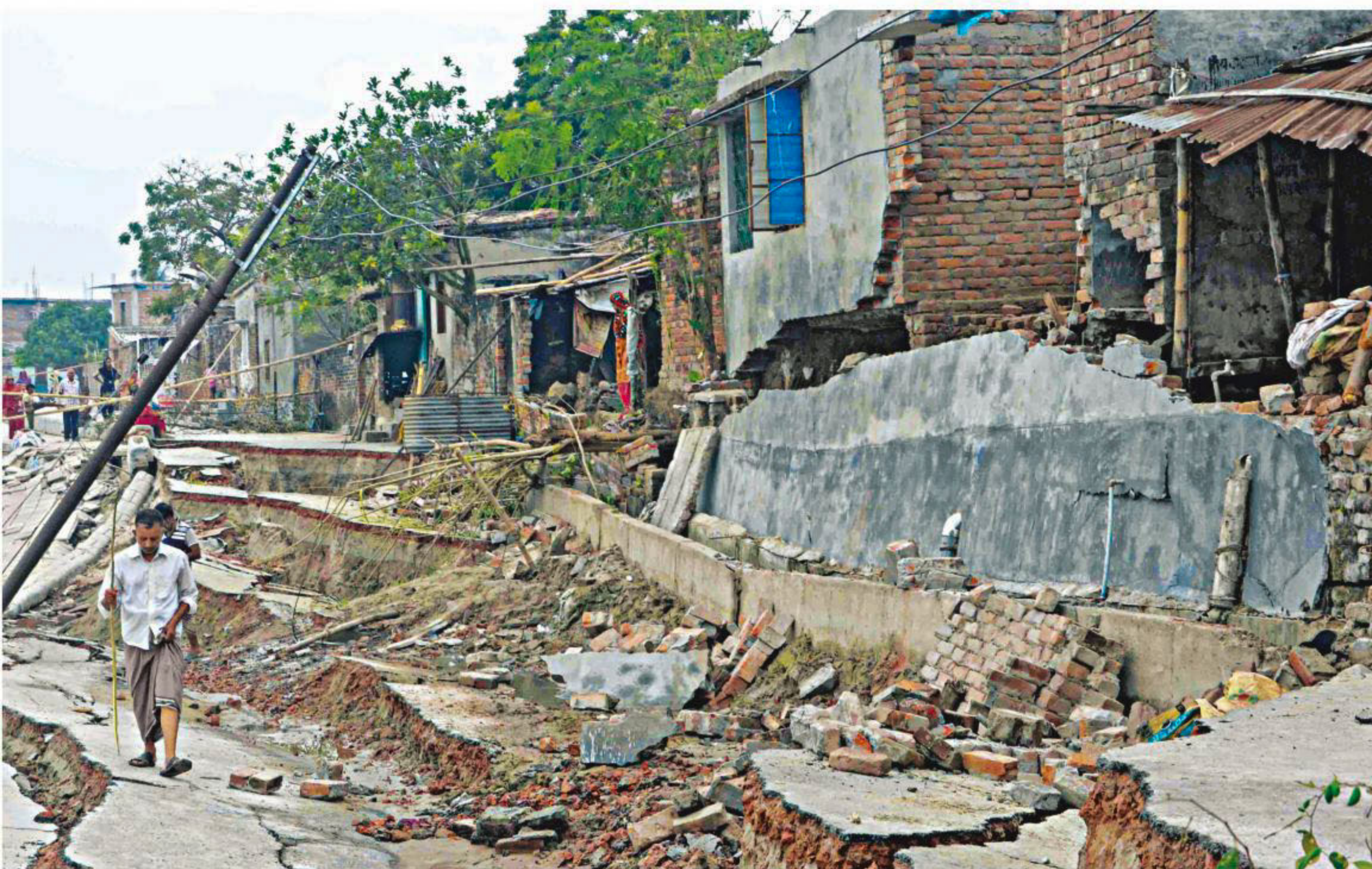
A person carefully walks on the subsided portion of the Padma river embankment in Rajshahi city's Shekher Chalk area yesterday. Some 60 meters of the land started subsiding from October 21 and went at least seven feet down damaging houses alongside the road.
