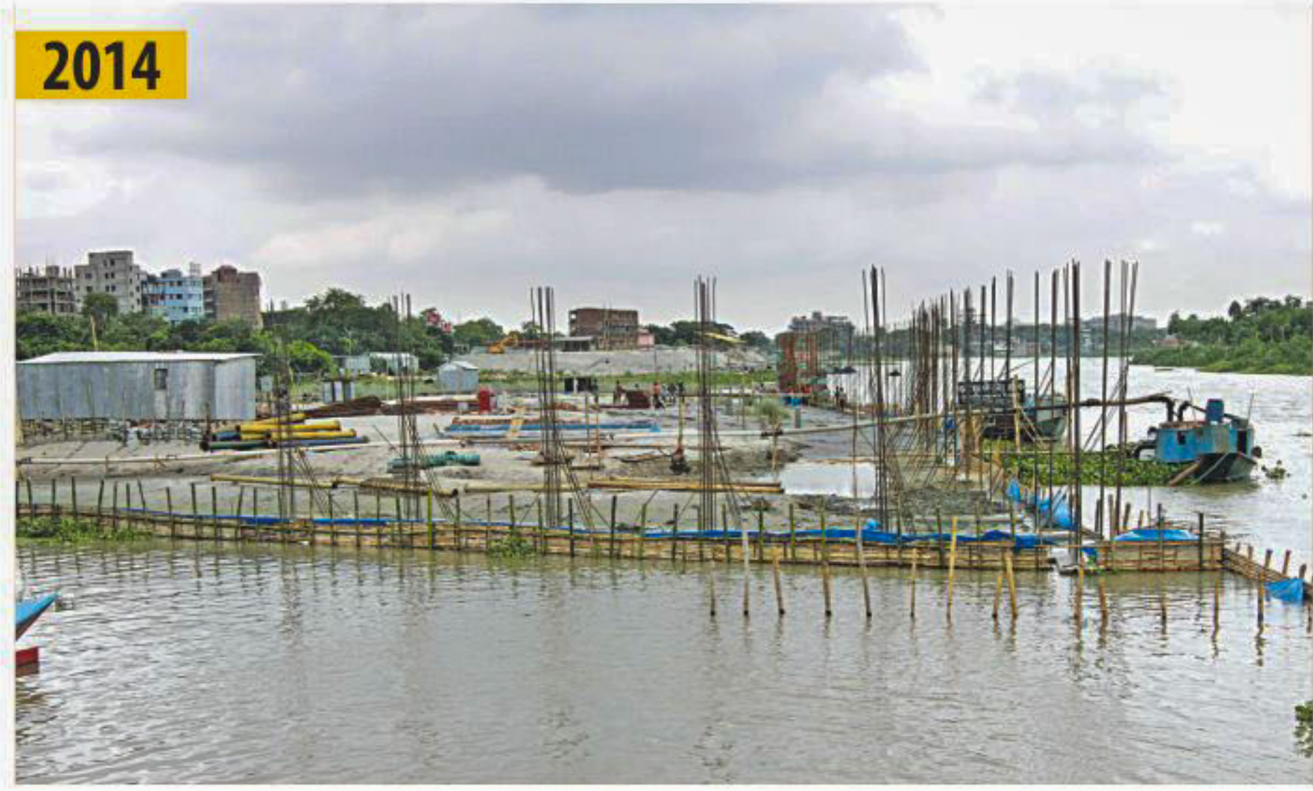
2014 Columns for a wall are being built on the newly made ground on the Turag near Kamarpara Bridge in Tongi.
