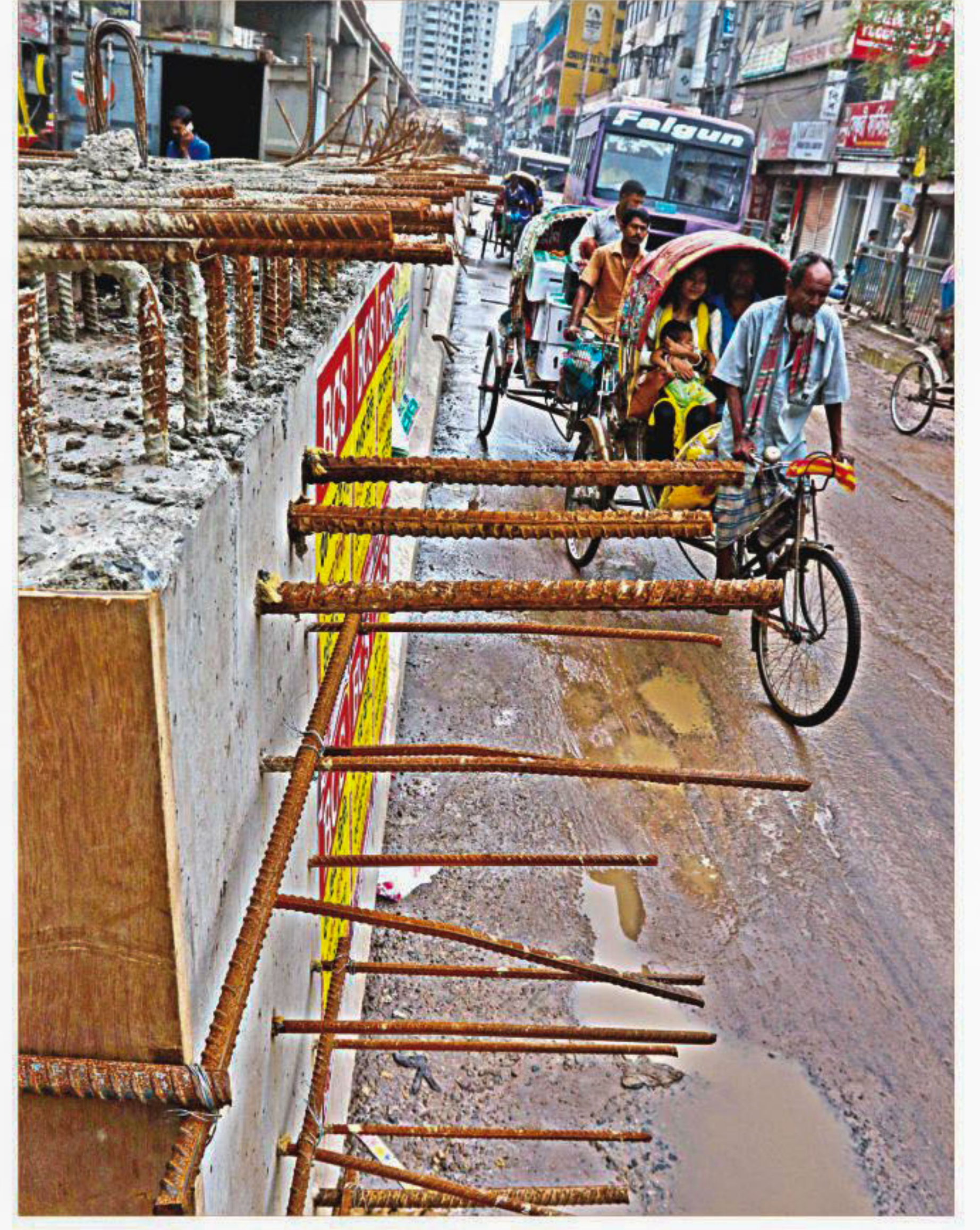
Rickshaws move gingerly past iron bars sticking out from a girder of the Moghbazar-Mouchak flyover on DIT Road near the Malibagh level crossing. The danger from this shoddy work seems to be overlooked in the daily hustle and bustle in this busy city. The photo was taken yesterday.
