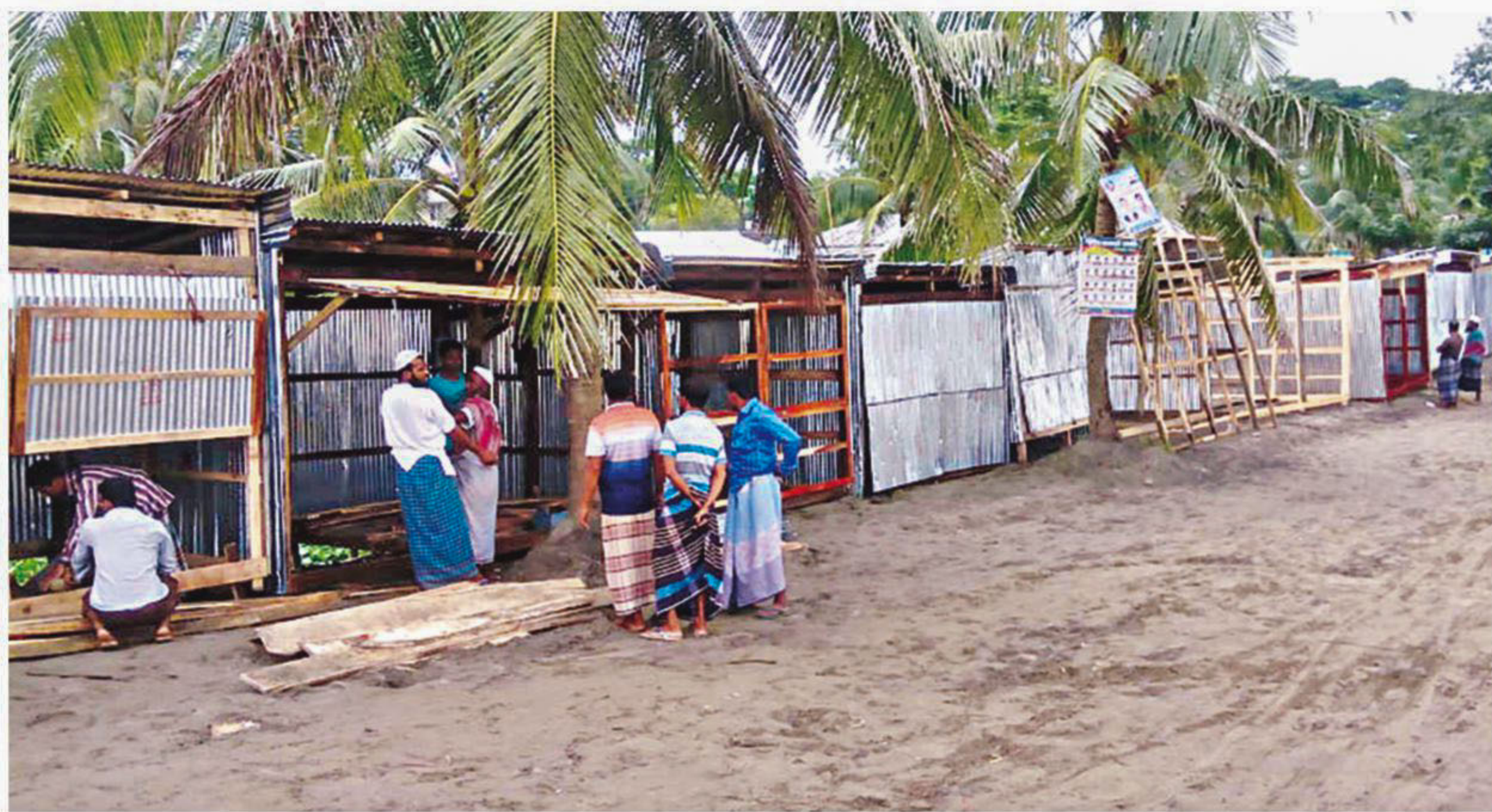
Structures go up on Kuakata beach ignoring a court order. The photo was taken yesterday.
