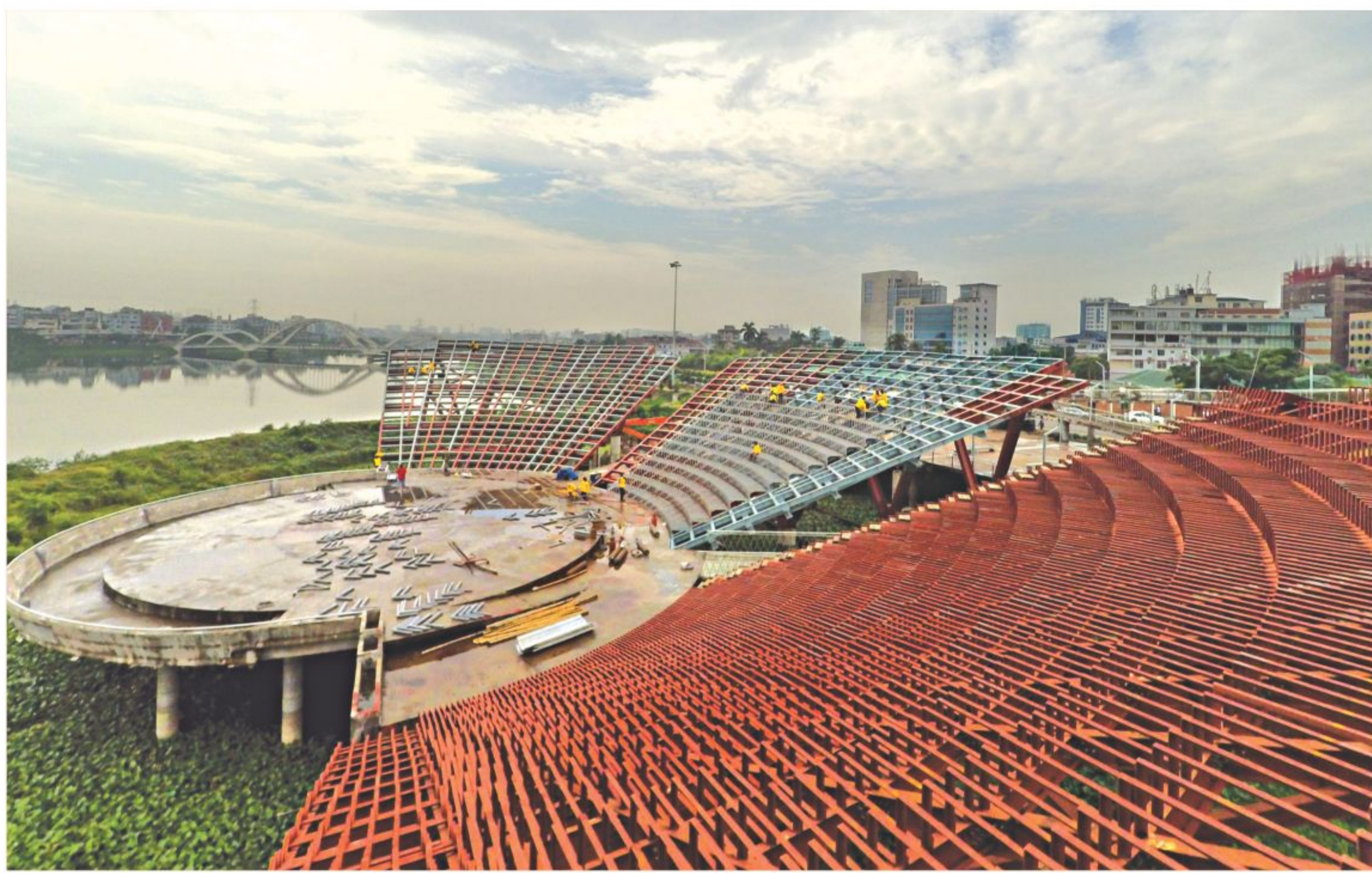
The construction of an international standard amphitheatre is underway at Hatirjheel in the city.
