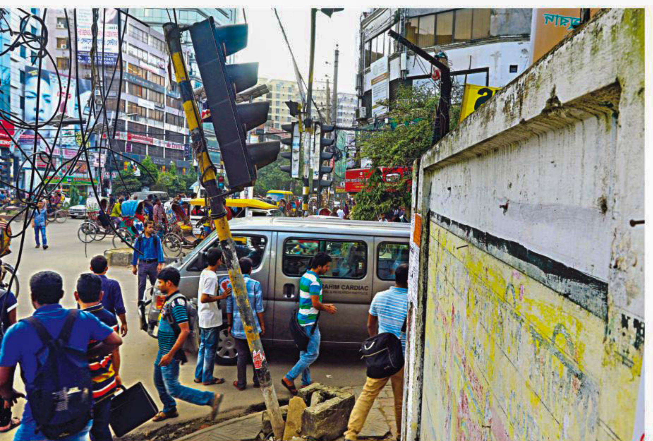
Pedestrians walk past a traffic signal post, leaning over the street, near the capital's Panthapath and Green Road intersection yesterday. The post has been left in this precarious position for a long time, which needs immediate intervention of the authorities concerned before any accident takes place. PHOTO: PALASH KHAN
