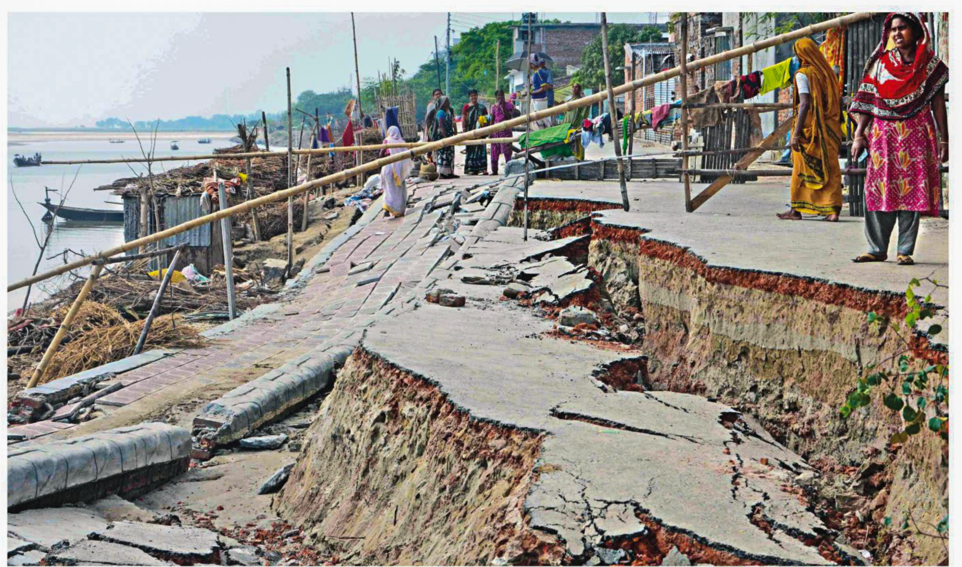
People look on bleakly at the subsided portion of a road over the Padma river embankment in Shekher Chalk area of Rajshahi city yesterday. Around 60 meters of the newly constructed road and walkway subsided on Friday night putting the near-by dwellers at risk. PHOTO: ANWAR ALI
