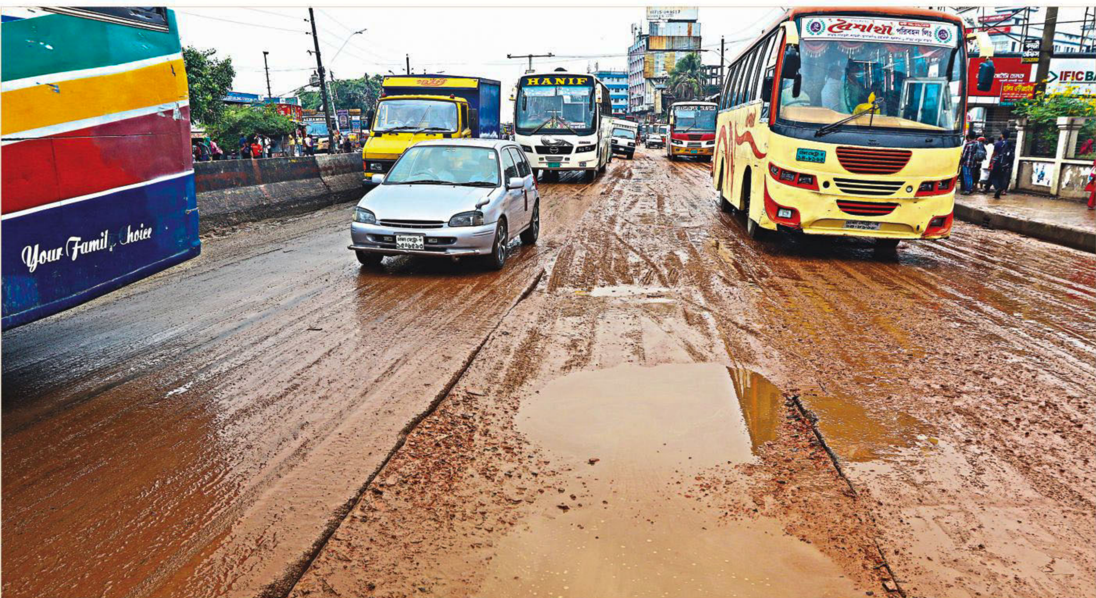
With a utility service provider digging up soil to install underground pipes for nearly a week, a light shower now suffices to turn the road into a completely muddy one, impeding vehicular movement and causing sufferings to pedestrians. The photo was taken in the capital's Gabtali bus stand area around noon yesterday. PHOTO: PALASH KHAN
