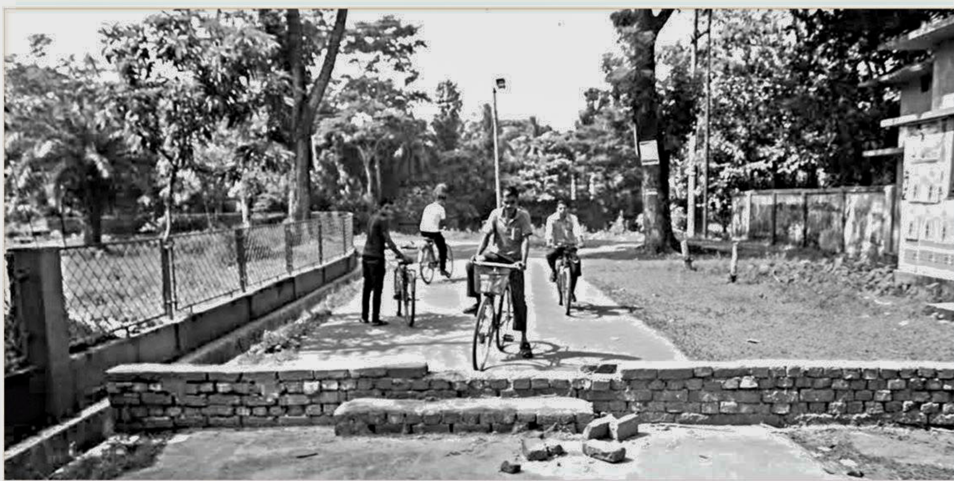
This wall was recently erected by Bangladesh Chhatra League activists on Sher-e-Bangla Medical College in Barisal "to prevent stalkers on motorcycles from preying on female students staying in a nearby hostel". The photo was taken recently.
