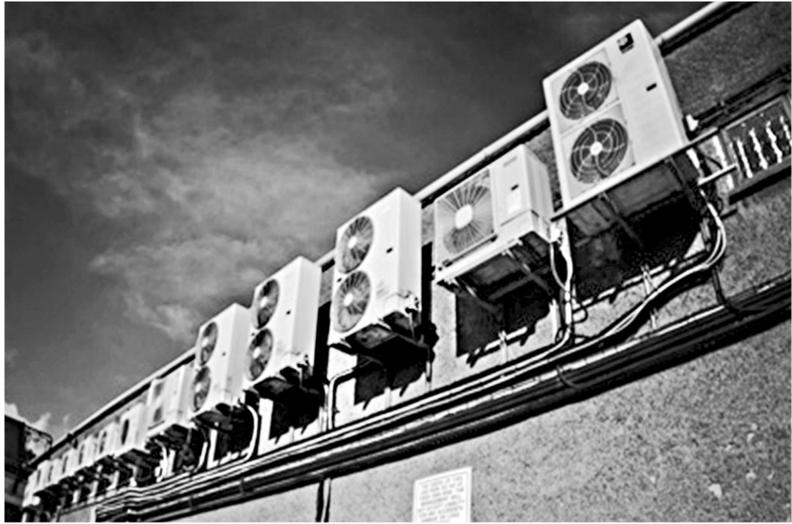
HFC gases are widely used in air conditioning units
