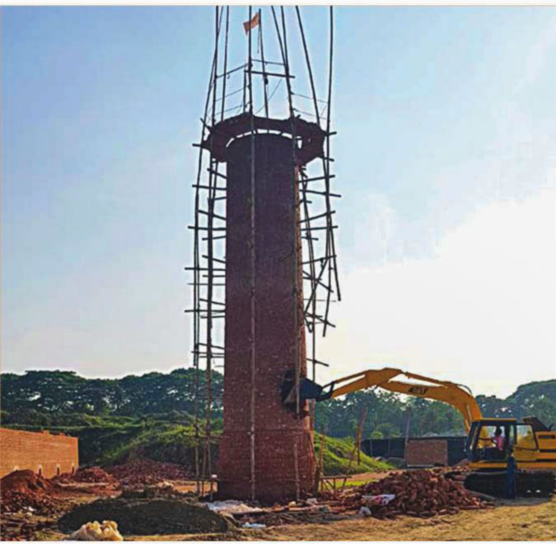
A bulldozer breaks the structure of MAF Brick Field-2 in Mojumdar Bazar area of Krishna Nagar union under Sadarpur upazila in Faridpur on Sunday as a mobile court of the district administration accompanied by the Directorate of Environment (DoE) officials conducted the operation. Earlier on October 19, The Daily Star ran a report on the harmful effect of the brick kiln set up on a farmland, without the permission of the DoE.
