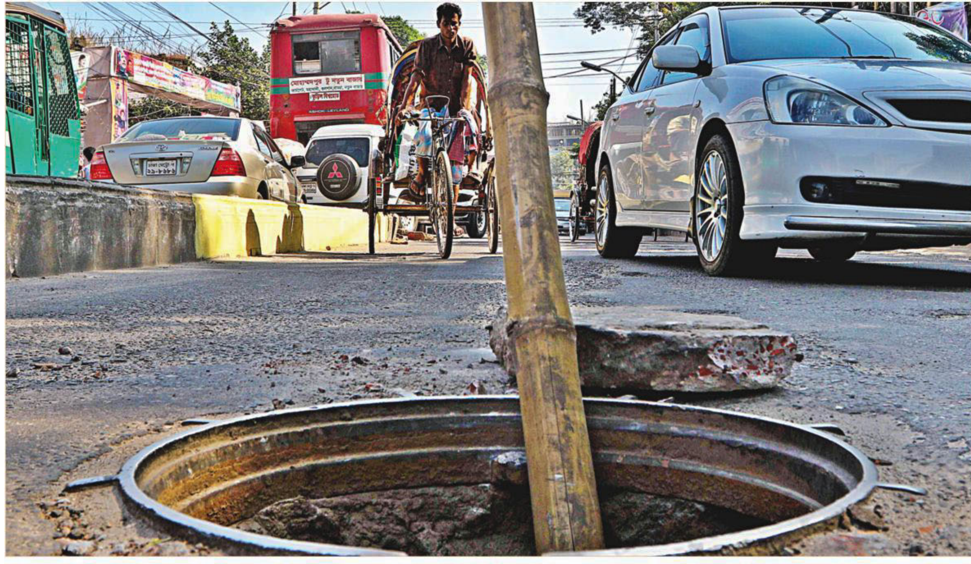
The bamboo pole in the open manhole warning oncoming vehicles not only is a signal for danger, but also is a symbol of the authorities' perpetual disregard for safety. It already has caused a few mishaps, and it is only a matter of time before a tragedy would befall the travellers. The photo was taken in Town Hall area in Mohammadpur yesterday. PHOTO: PRABIR DAS
