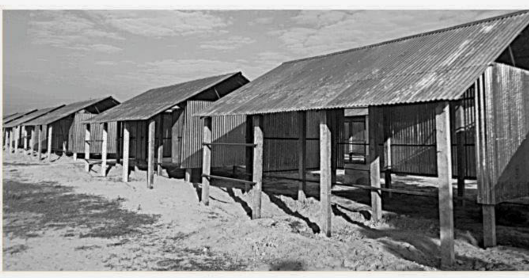
An under-construction cluster village for the homeless people at Jorgachha union in Sonatola upazila of Bogra. PHOTO: STAR
