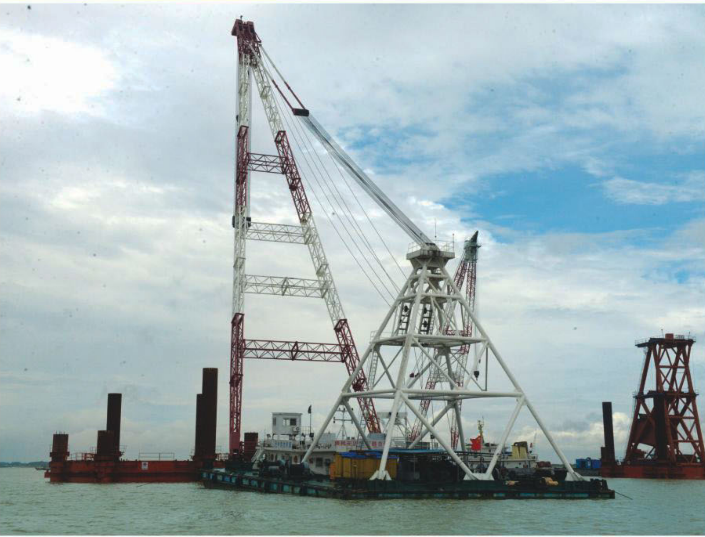
Construction site of the Padma bridge on the outskirts of Dhaka, capital of Bangladesh. In June 2014, the Bangladeshi government awarded China Major Bridge Engineering Company Limited a 1.55-billion-U.S. dollar contract to build core structure of the Padma bridge project which is to be completed in four years. (Xinhua/Shariful Islam)
