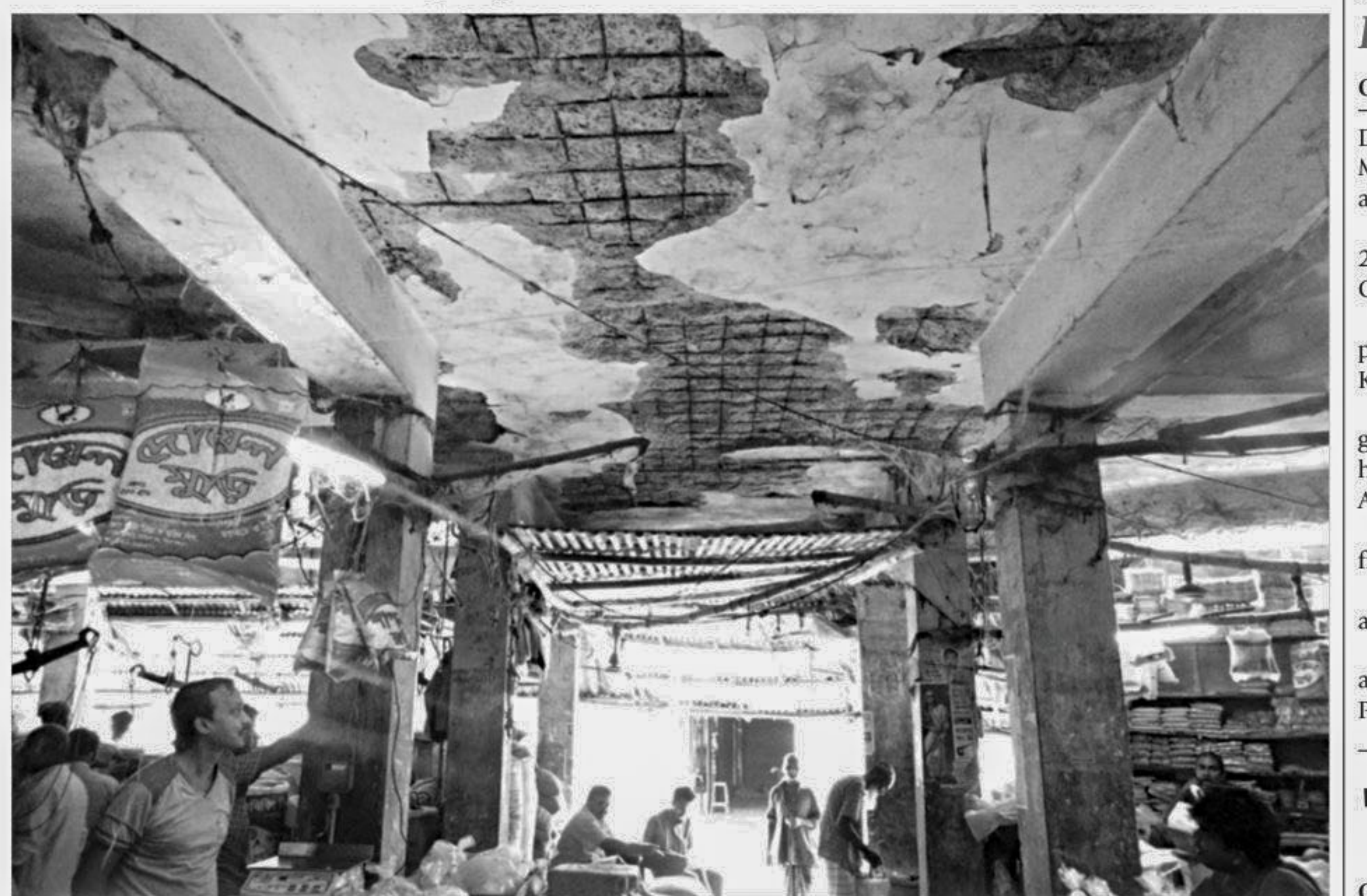
The ceiling of the Kaliganj covered market in Jhenidah is in a shocking state of repair, posing a life risk to traders and shoppers every day.
