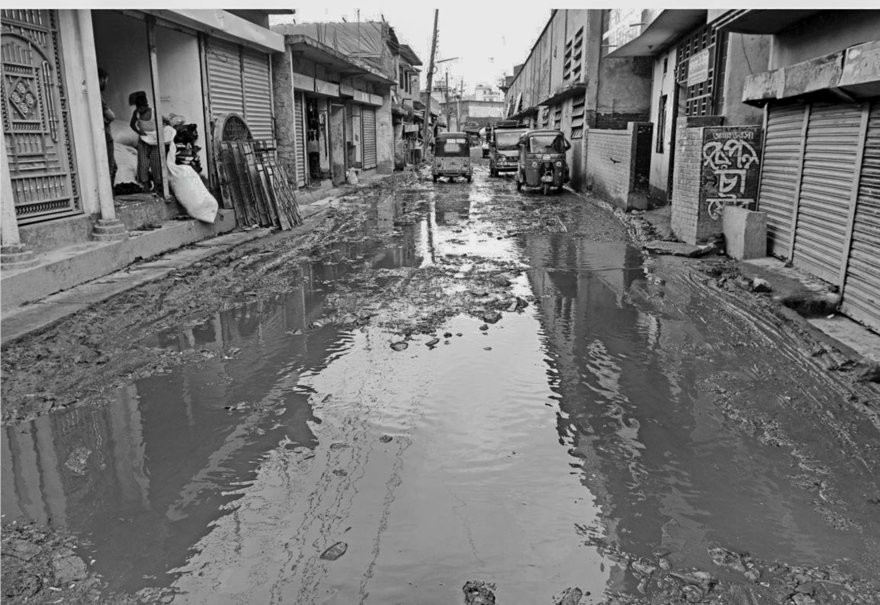
Rainwater stagnates on the dilapidated Kalunagar road in the capital's Hazaribagh due to a poor drainage system, impeding vehicular movement. The photo was taken yesterday.
