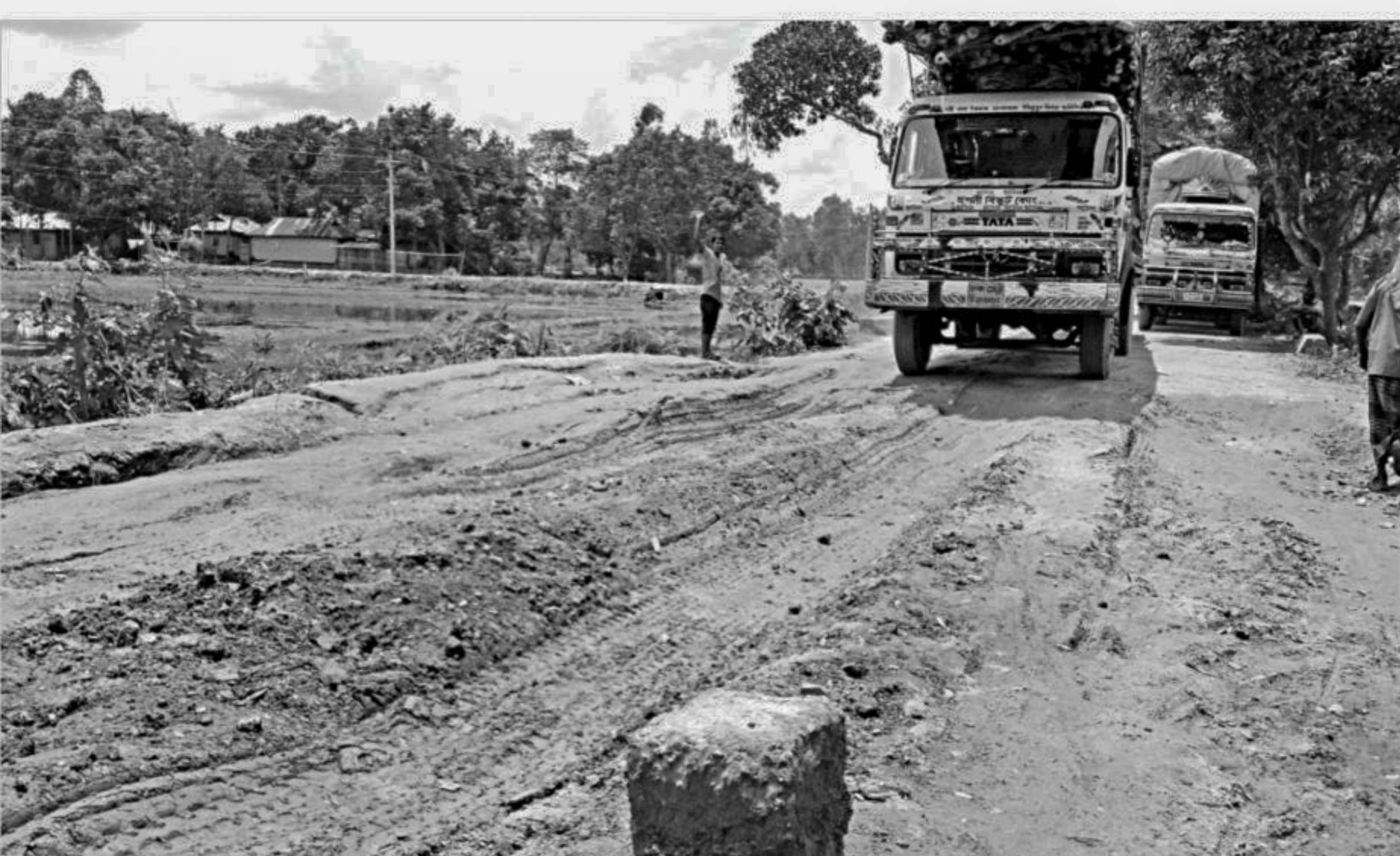
Awful condition of the five and a half kilometre Mahendranagar-Barbari road that connects the Lalmonirhat district headquarters with other upazilas. The photo was taken a few days ago.
