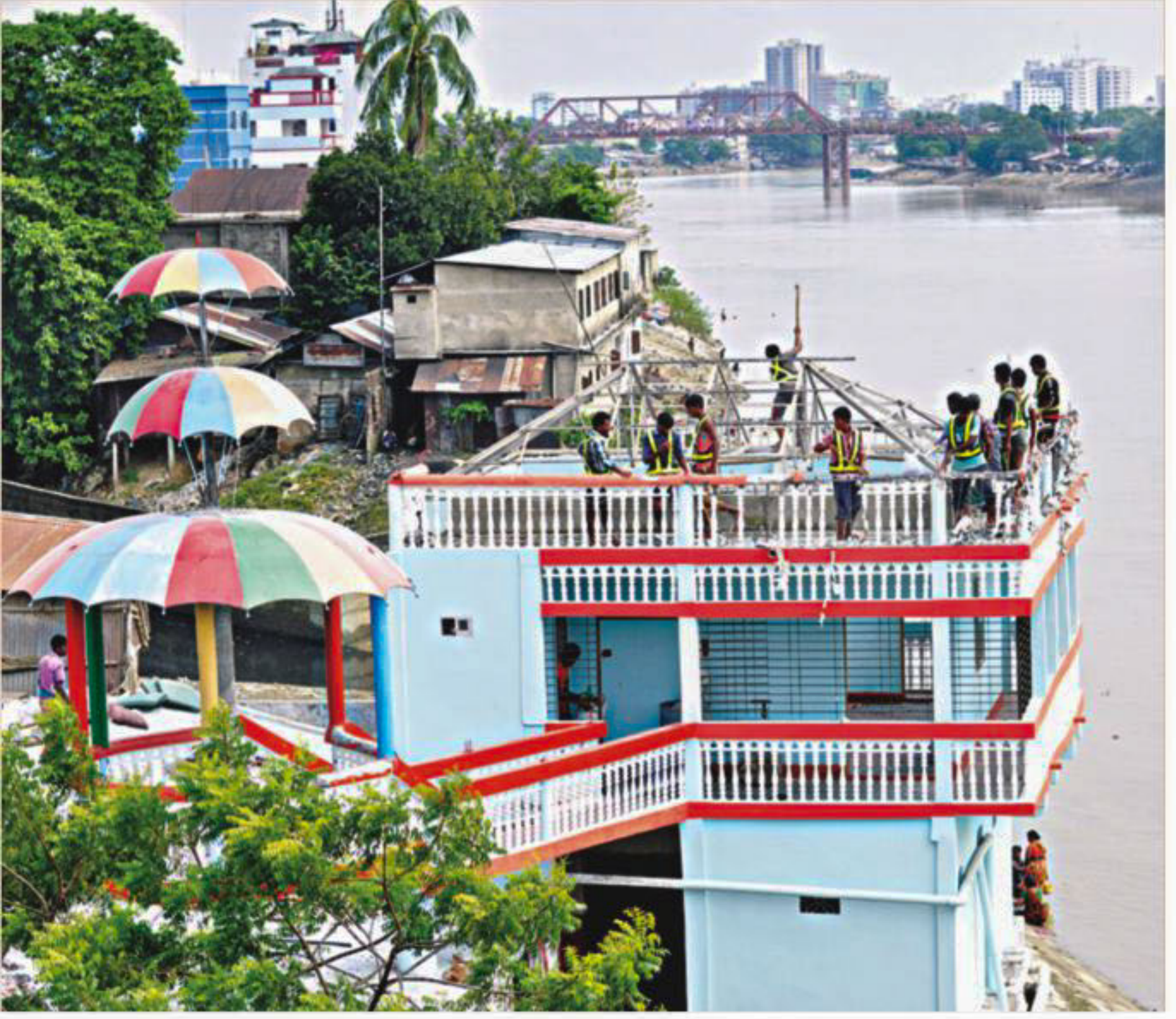
Workers, under the authority of Sylhet District Administration, dismantle a portion of the recently constructed building, which housed around eight restrooms for the fish traders of the area, on the eastern side of the Surma river yesterday. The Daily Star also published two reports on September 10 and 30, highlighting how waste was directly being released into the river from those.
