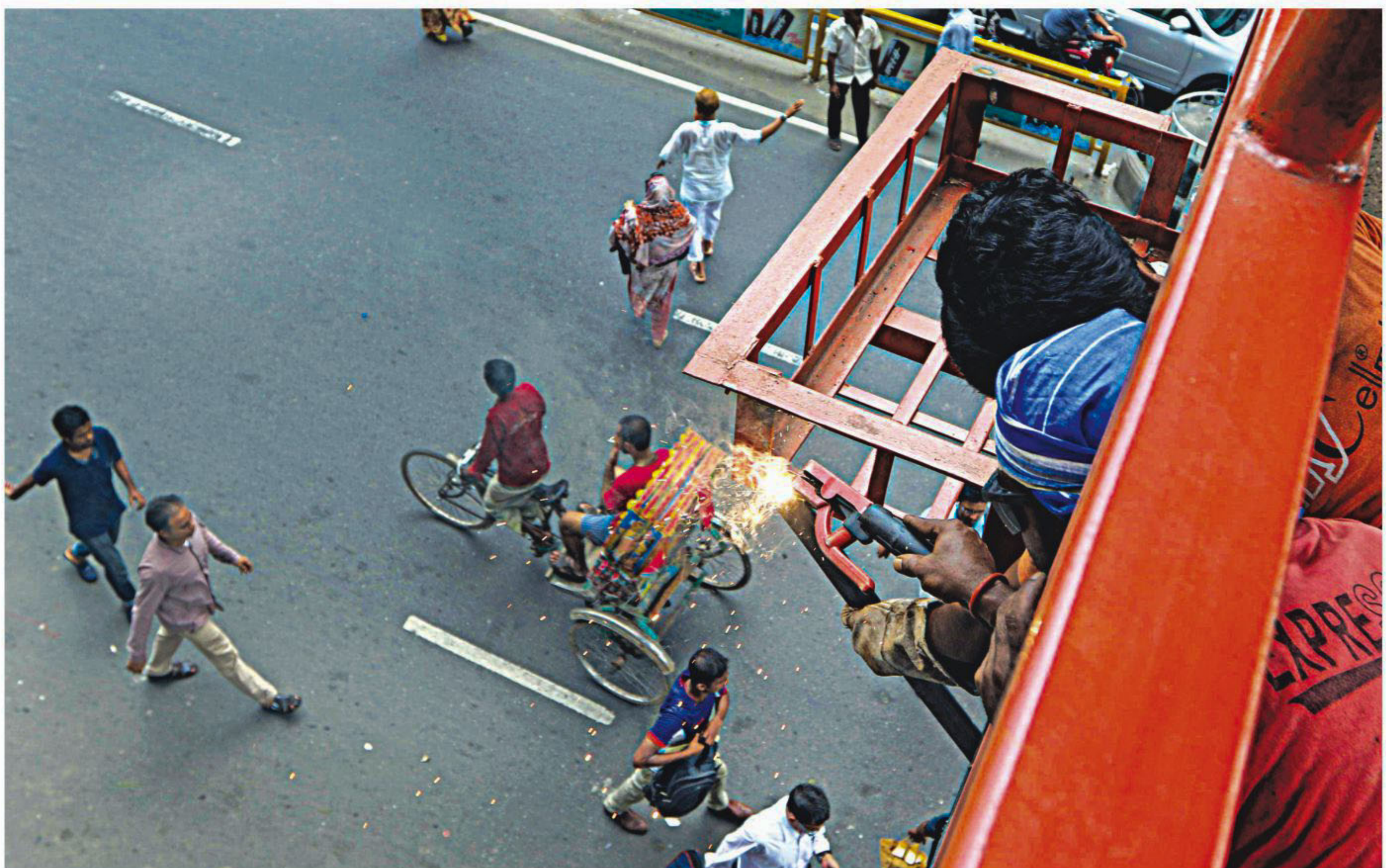
Without taking any safety precautions, two workers weld metal frames on a footbridge in the capital's Shahbagh area. Pieces of metal may fall off during the welding, and injure pedestrians and damage vehicles. The photo was taken around noon yesterday.
