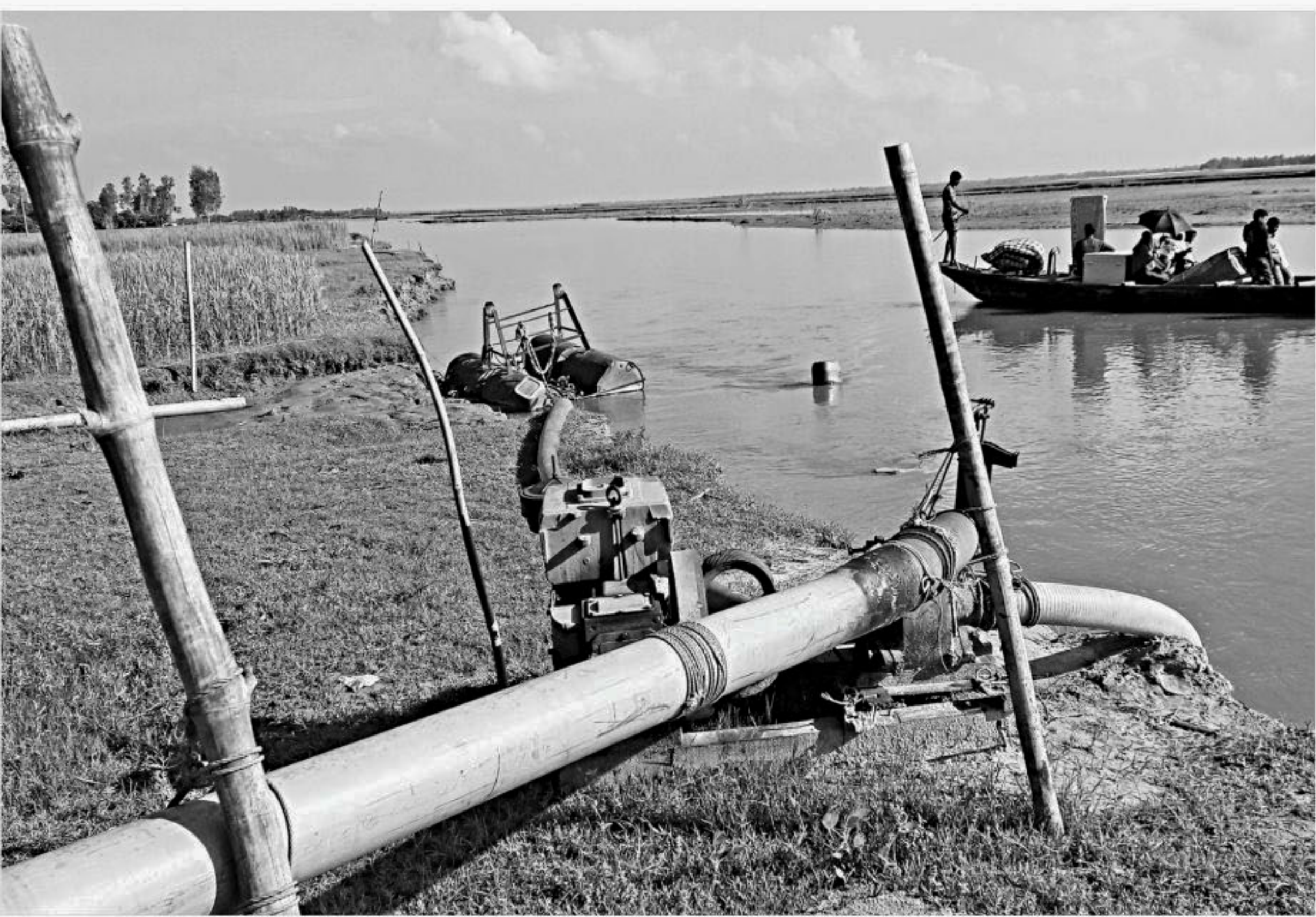
Illegal sand lifting from the Teesta river has increased erosion, which is devouring croplands and homesteads in Char Gokunda village in Gokunda union under Lalmonirhat Sadar upazila. The photo was taken recently.
