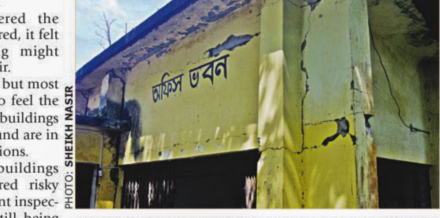
One of the many derelict buildings of the government's poultry farm office in Tilagarh of Sylhet city.
