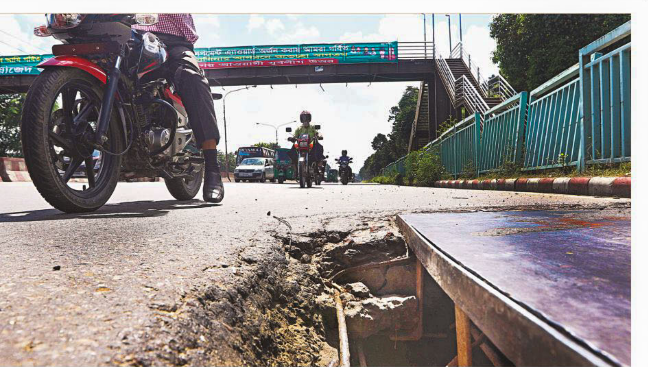
With asphalt around this underground utility cable pocket getting removed, it is now contributing to frequent traffic accidents in the area, particularly at night when vehicles' drivers and commuters overlook the pocket. Locals say a number of motorbike riders have fallen victim of deadly accidents in the last few days due to it. The photo was taken on the airport road in the capital's Kawla recently. PHOTO: PRABIR DAS
