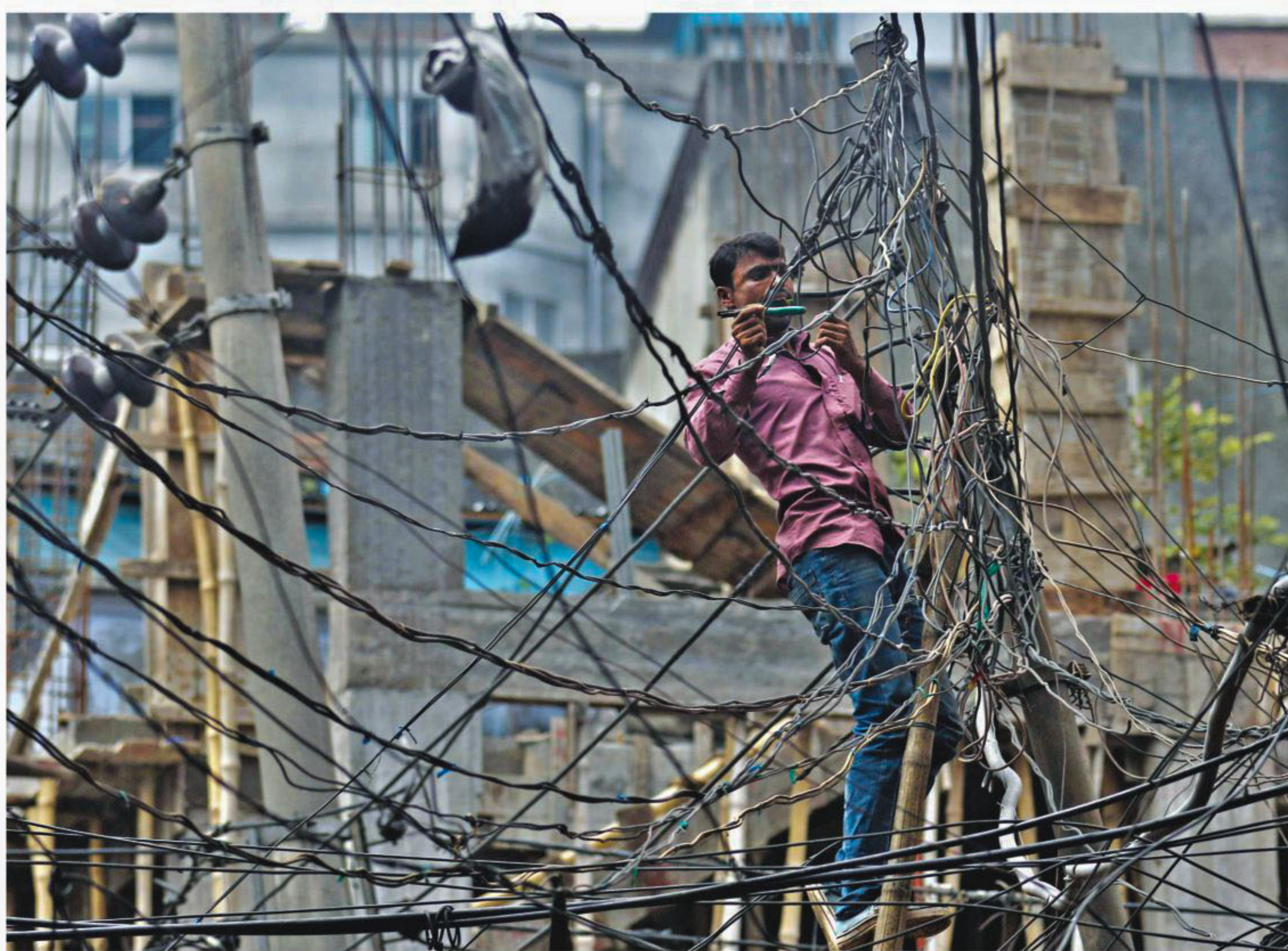
With no safety gears on, a power technician works in the maze of power, cable TV and internet cables on Northbrook Hall Road in Bangla Bazar of Old Dhaka yesterday.
