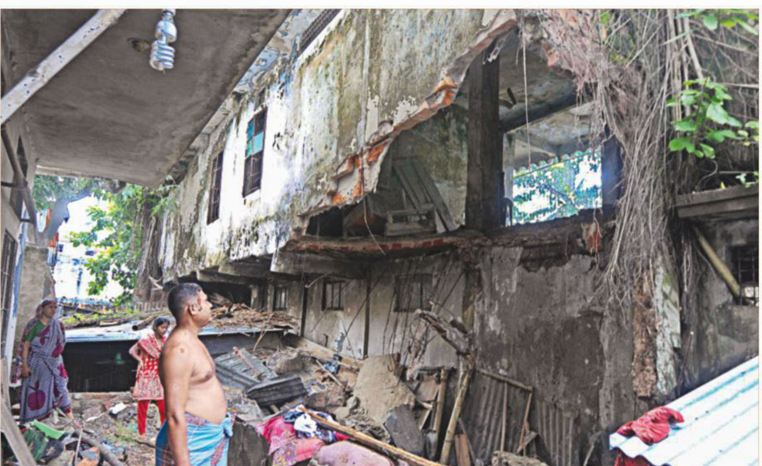
A man stares at the portion of an abandoned building in Mirpur's Shah Ali area, which collapsed on a tin-shade house around 3:00am yesterday killing a teenage girl and injuring a minor boy. The abandoned building belonged to the department of social services, who used it as a shelter and later shifted following its dilapidated condition.
