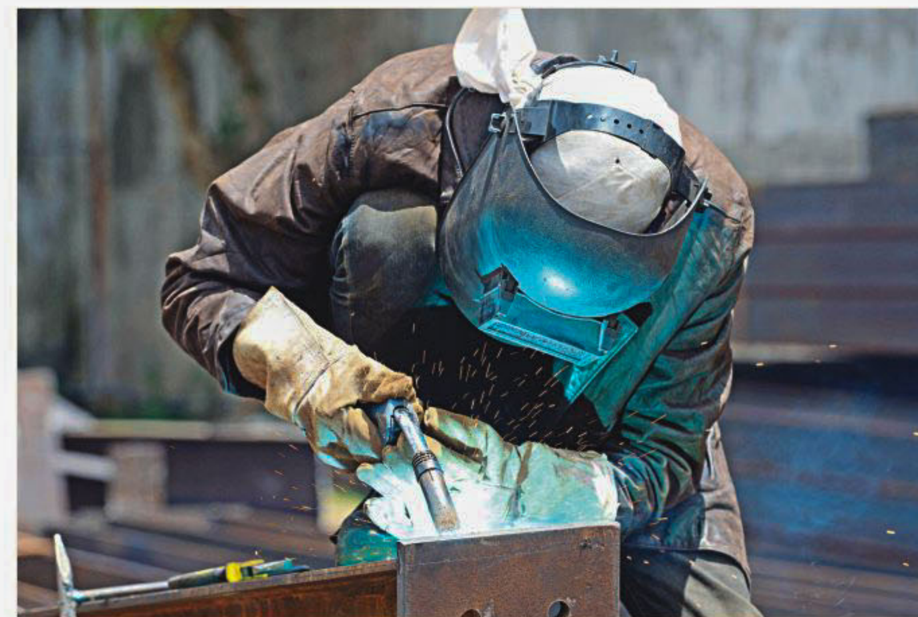
A Sri Lankan ironworker welds material at a building site in Colombo on Sunday. Sri Lanka's unity government faced opposition from business leaders and the opposition to proposals to increase VAT by 4 percent, from 11 percent to 15 percent. Despite Cabinet assurances the increase is a temporary measure, an IMF mission visiting the country said, "It will be a source to support revenue targets and we do not see it as a temporary measure."
