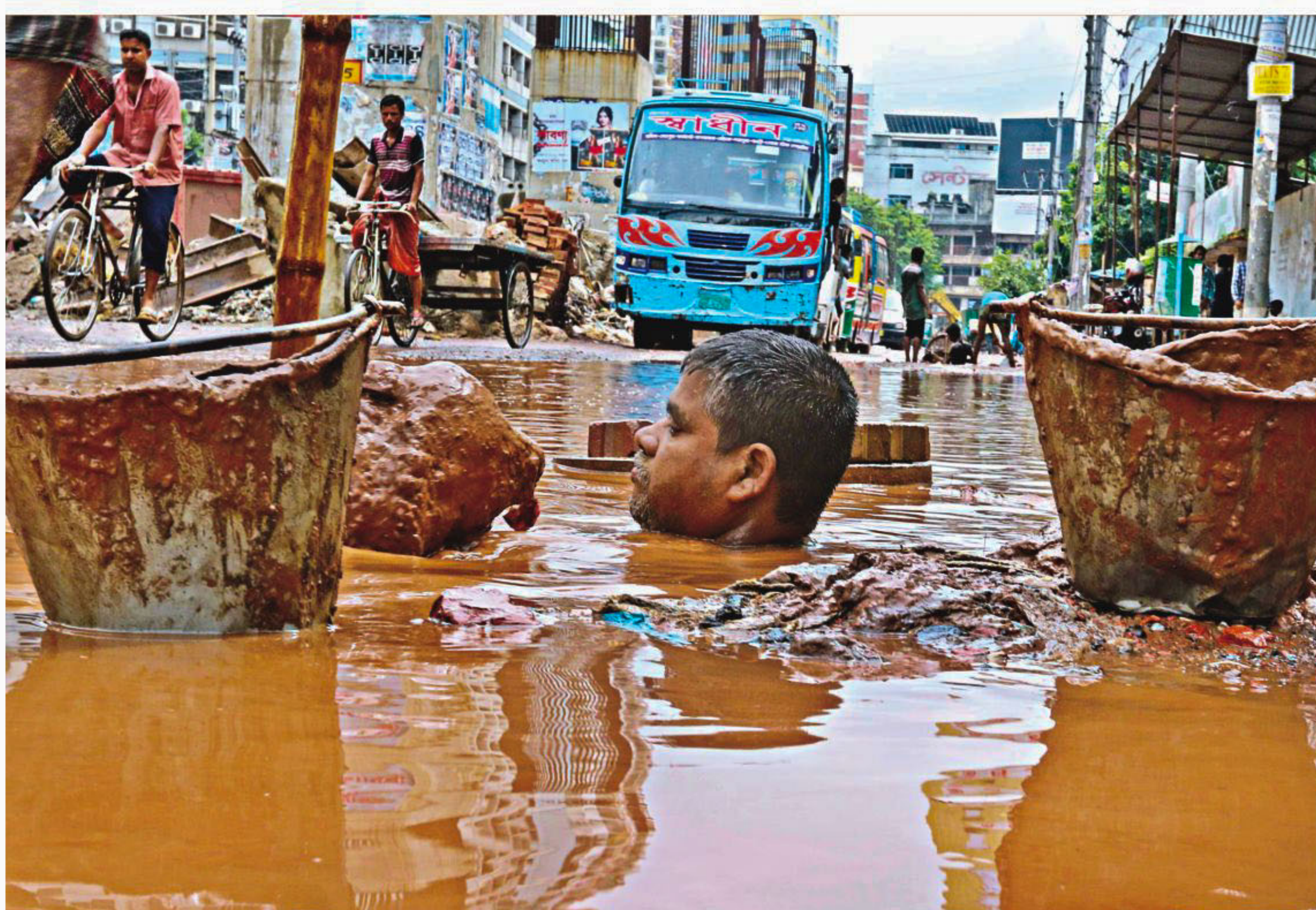
Without any safety gear, a worker cleaning a manhole near the Moghbazar-Mouchak flyover after yesterday's downpour. Mud and debris from the construction work of the flyover often clog the drainage system there, inundating the street. The man could easily be run over by a vehicle or even drown. The photo was taken around 1:30pm at Pashchim Malibagh.
