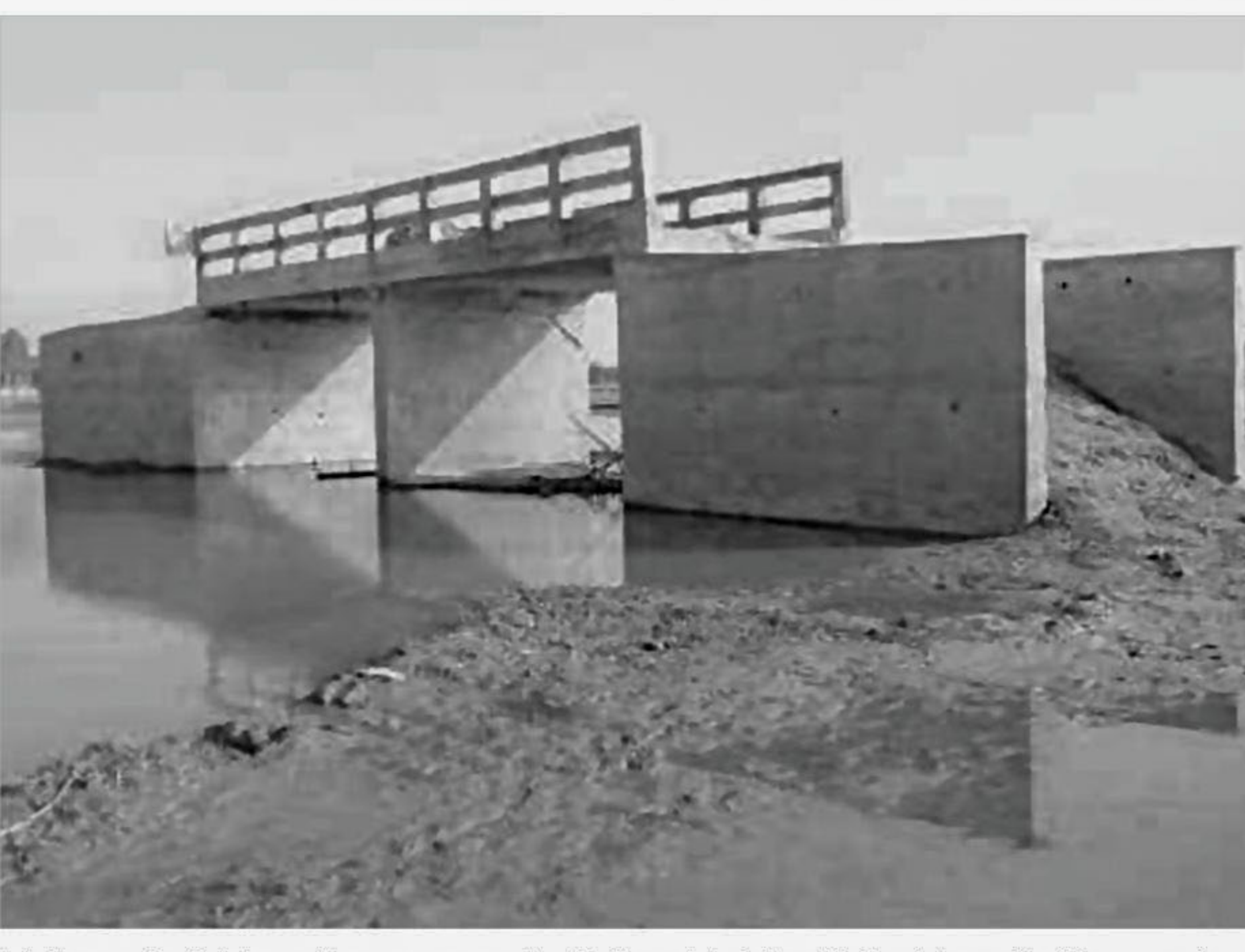
A bridge constructed six months ago over a canal at Khatiamari-Amtoli road in Sonatola upazila of Bogra remains a mockery for locals as connecting roads are yet to be constructed to make it usable. PHOTO: STAR
