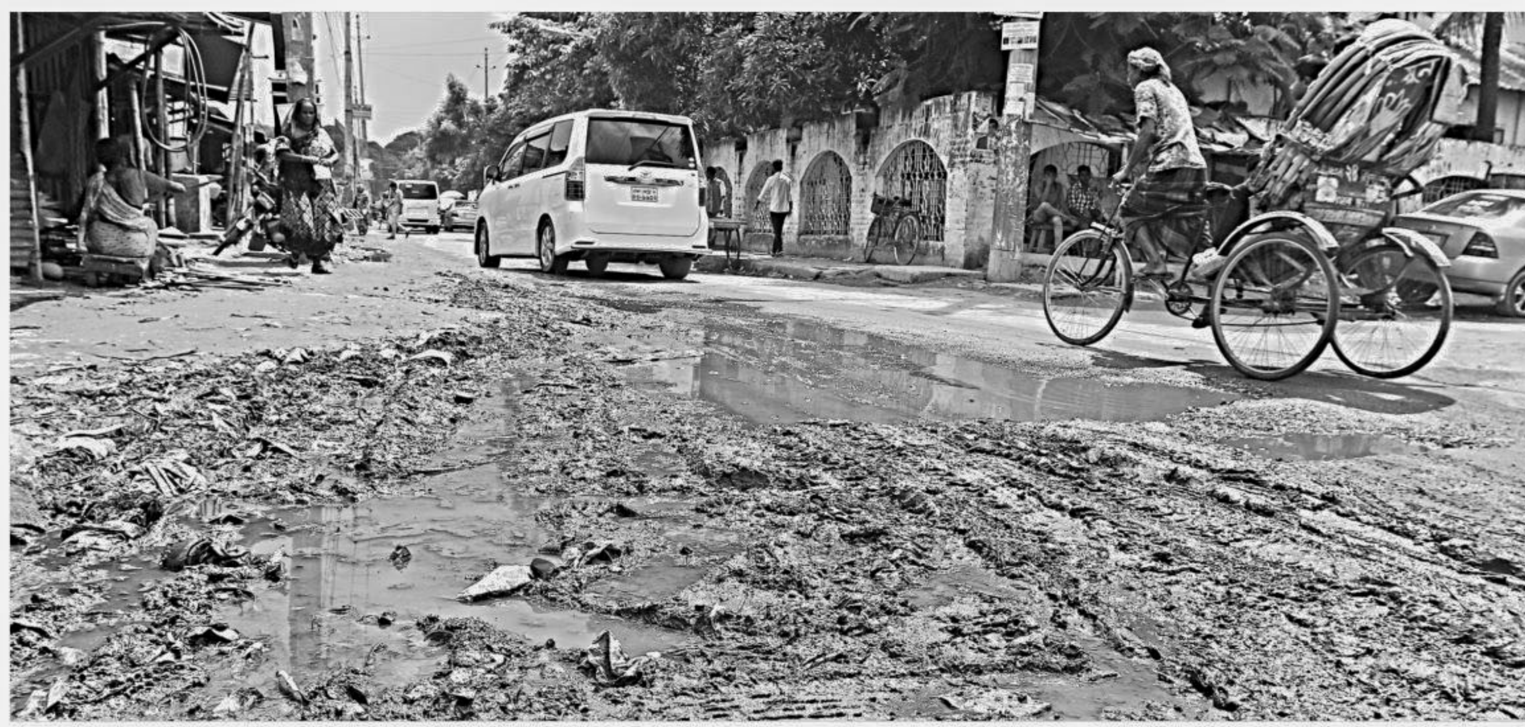
As the bitumen surface of this major portion of a road before Islamic Foundation in Dhaka's Agargaon has got completely damaged and eventually rainwater made it muddy, it mostly remains unused. The photo was taken yesterday.
