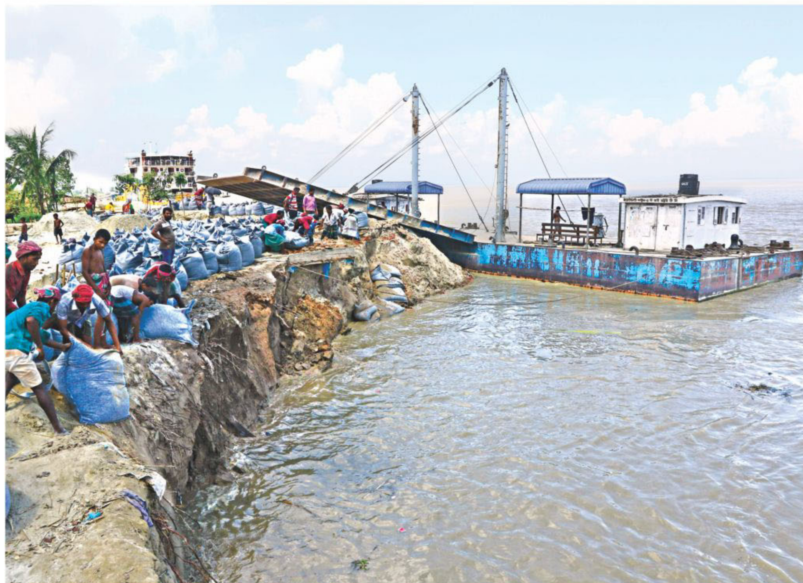
Workers dump sandbags to prevent erosion by the mighty Padma near a landing station of Daulatdia ferry terminal. Two of the four landing stations at the terminal are out of service as the river has devoured its bank near the pontoons, severely disrupting ferry service between Paturia and Daulatdia.
