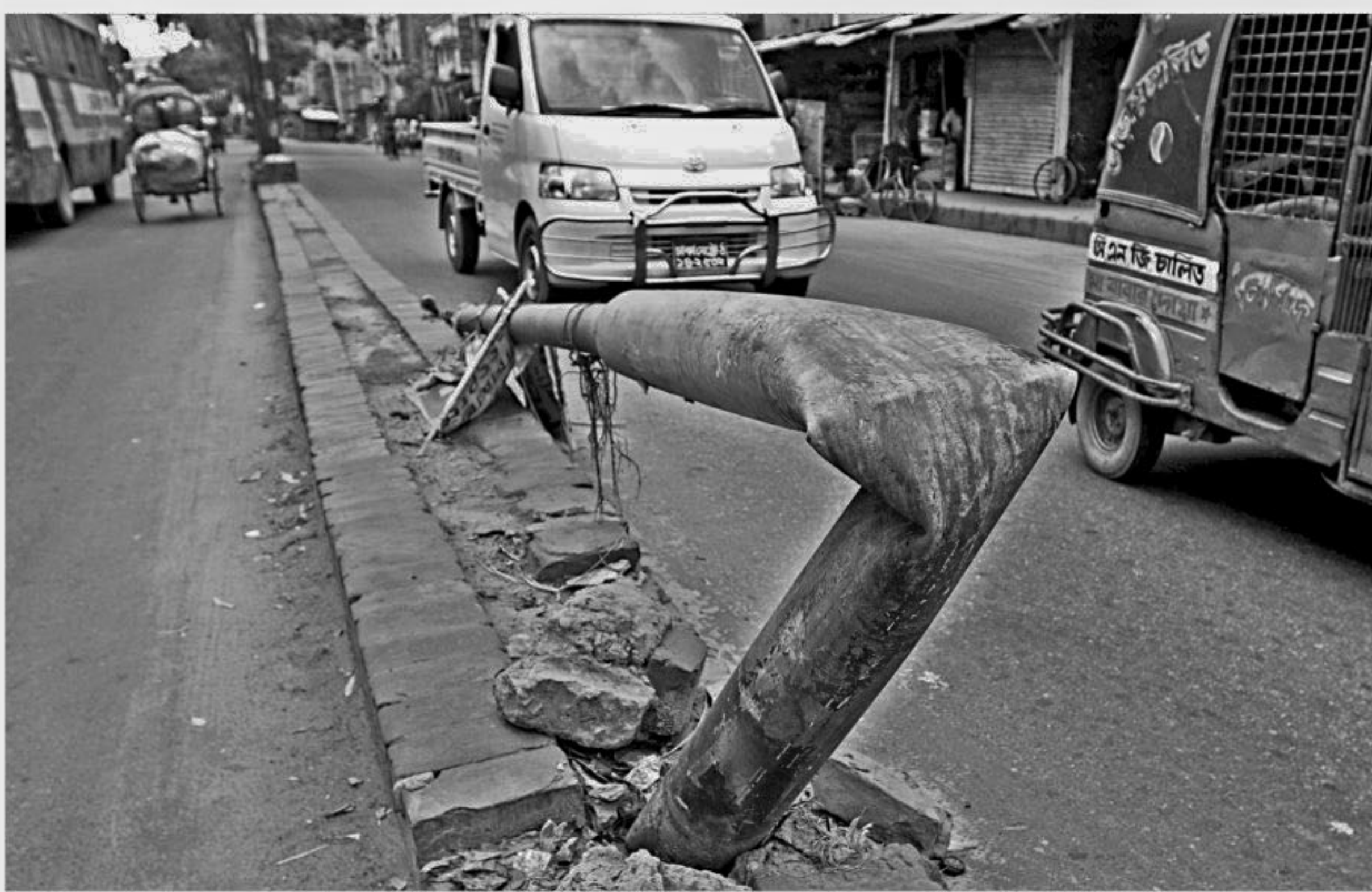
The wrecked utility pole has been left in this state for quite a long time, which might cause a fatal accident anytime. The photo was taken at Dholpur of Jatrabari in the capital yesterday.
