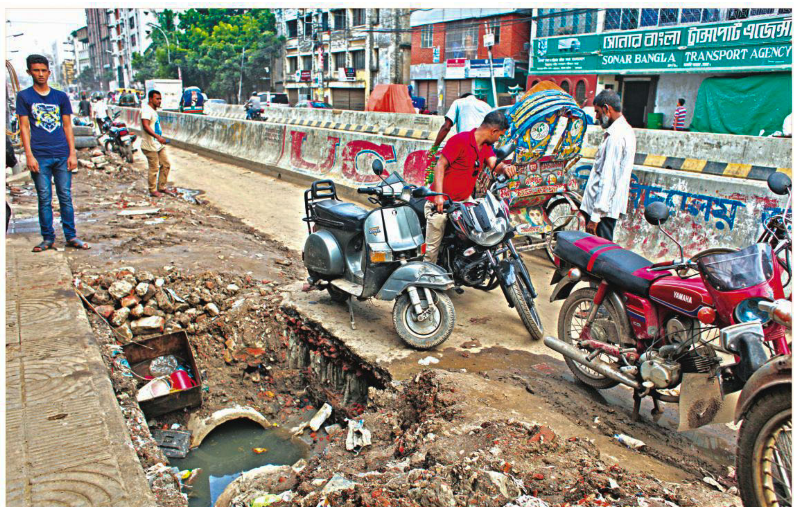
Digging for repairment has rendered the road near the Medical Mor in the capital's Bakshi Bazar almost unusable because it leaves barely any space for vehicles. It was not just one day or two that the commuters and pedestrians had to endure, the road has been left in this state for two weeks. The photo was taken yesterday.
