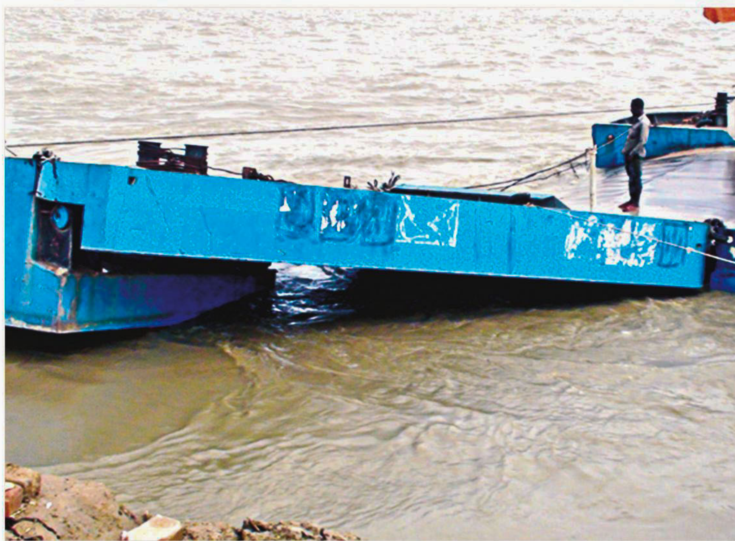
The dislodged pontoon of a ferry landing station at Daulatdia Ferry Terminal yesterday. The Padma devoured a part of its bank at Daulatdia of Rajbari, causing disruption to ferry services on Paturia-Daulatdia route.
