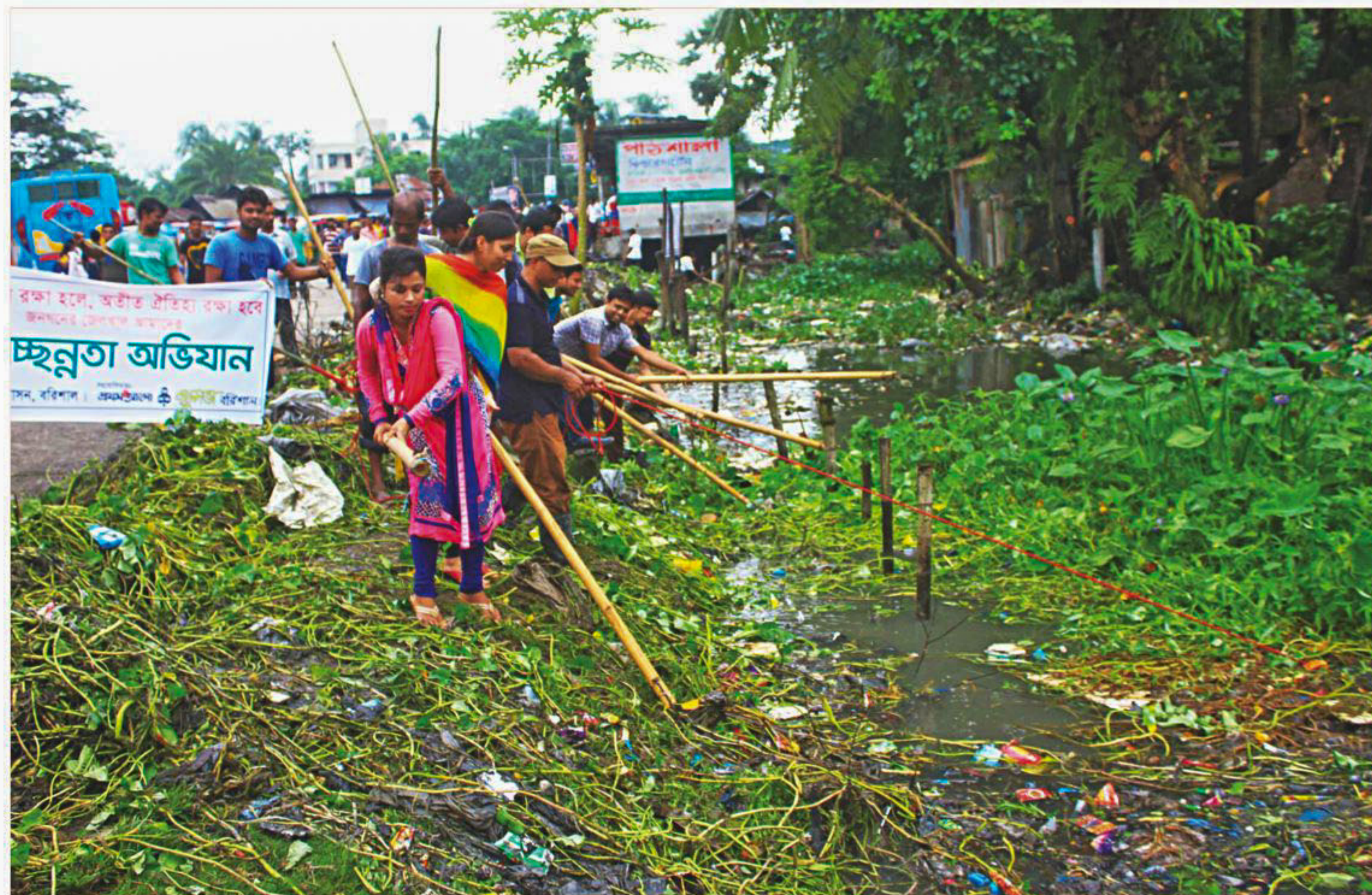
As part of a move to save Barisal city's Jail Khal from encroachment, people join a drive conducted by the district administration to clean the canal yesterday. In the last four months, the authorities demolished more than 100 illegal structures on its banks. PHOTO: ARIFUR RAHMAN
