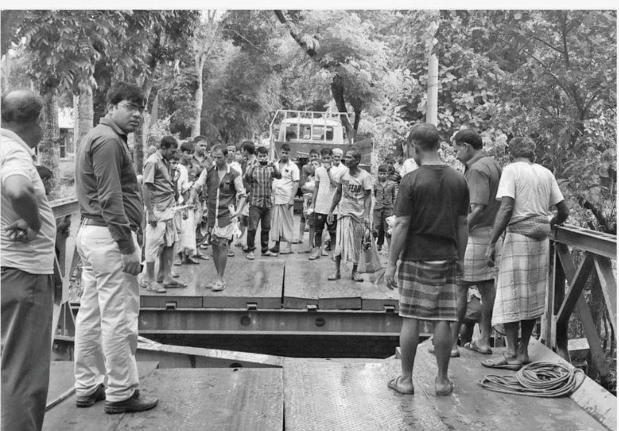
Road communications between Bandarban and Rangamati remain snapped following the collapse of a Bailey bridge in Sadar upazila of Bandarban on Wednesday.
