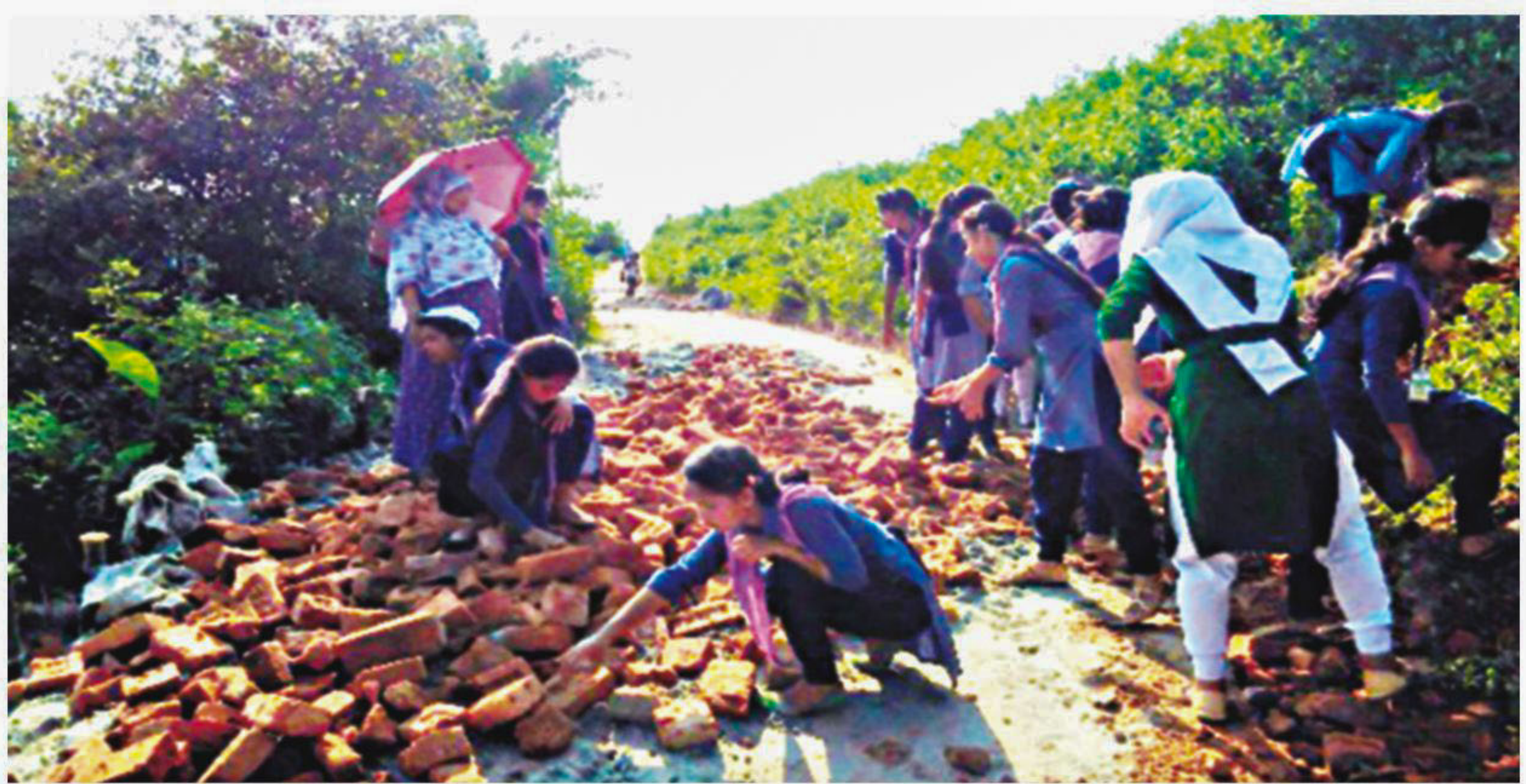
Students of Dhamshor Halimunnesa Chowdhurani Memorial Girls High School repairing a road on their own in Bhaluka upazila of Mymensingh on Monday.
