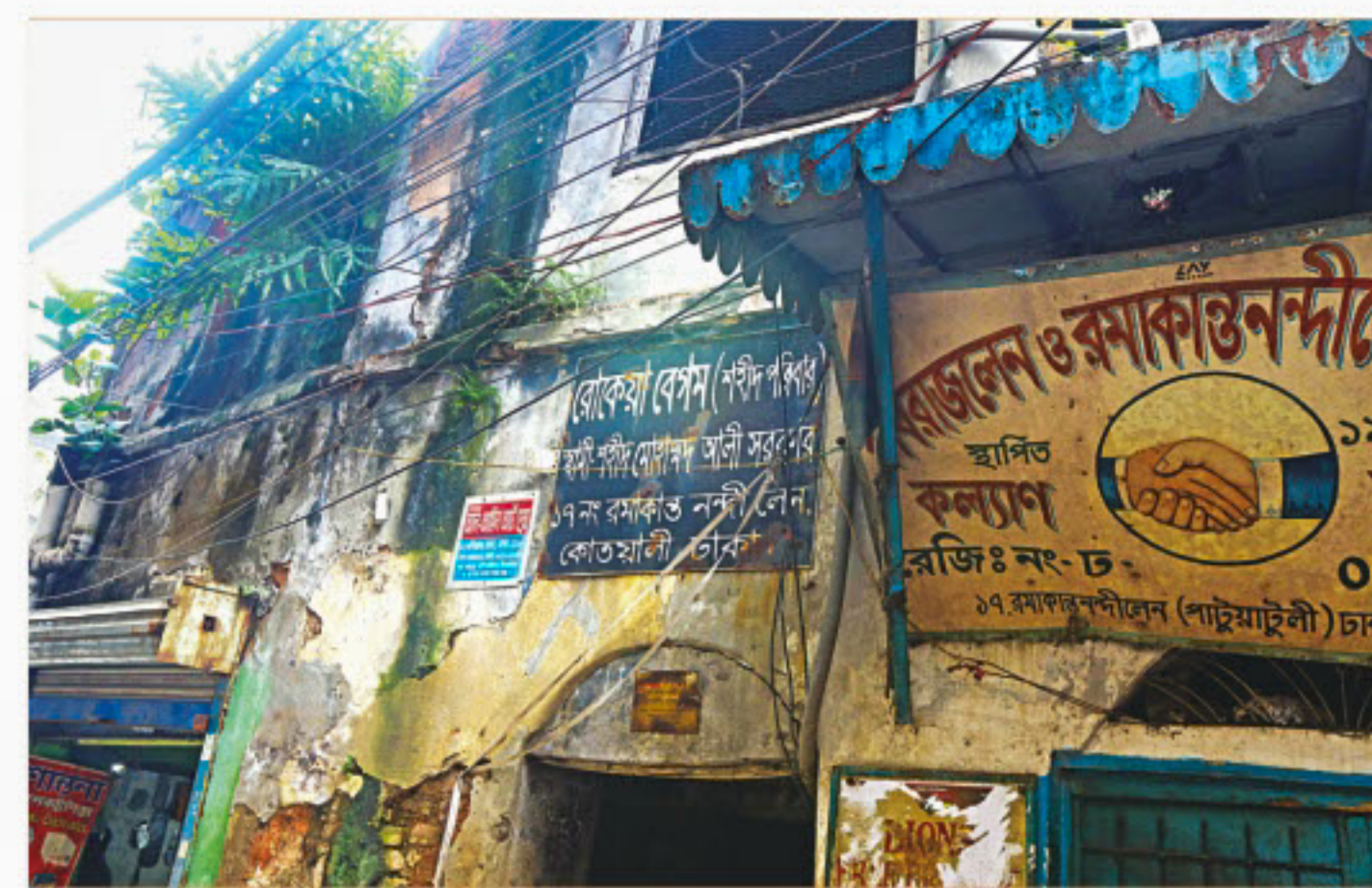
3. A family claiming to be of a Liberation War martyr has taken over Shaheed Azmal Hossain Hall.
