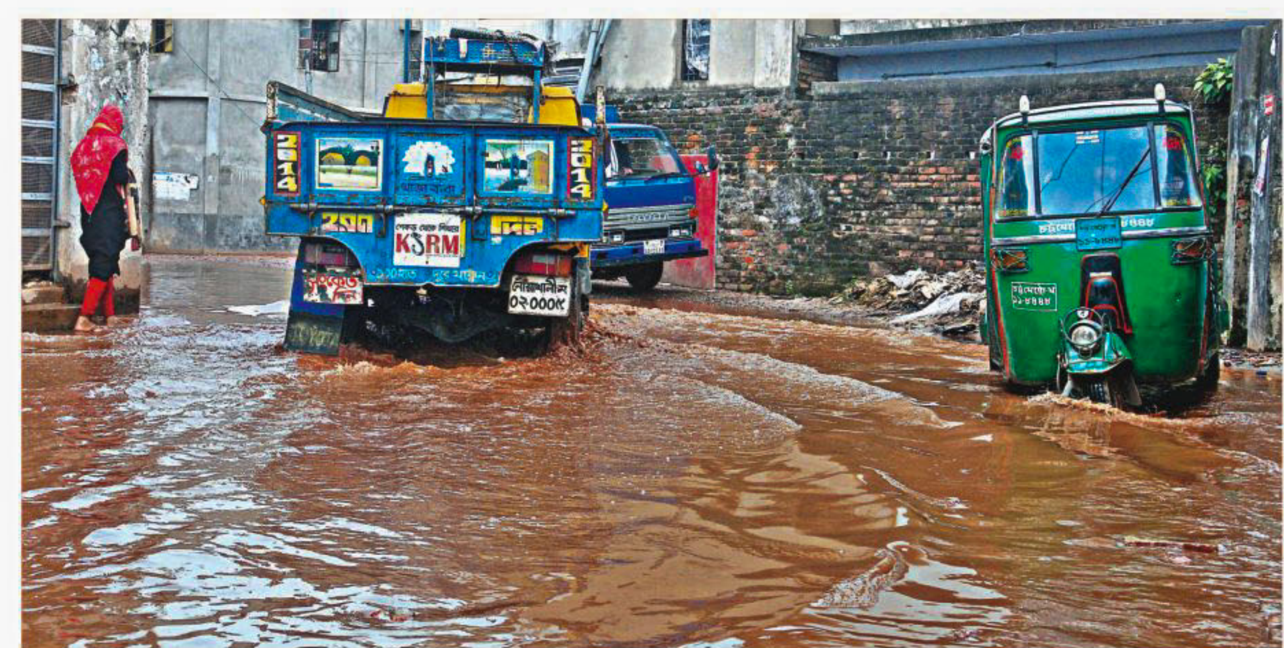
Sewerage water floods a road in Kalurghat BSCIC industrial area of Chittagong city, washing away what remains of its asphalt surface. Due to movement of heavy vehicles, the road is already in bad shape, and the dirty water has compounded the problem. However, the situation has remained unchanged for the last few months, while people keep suffering. The photo was taken Saturday.
