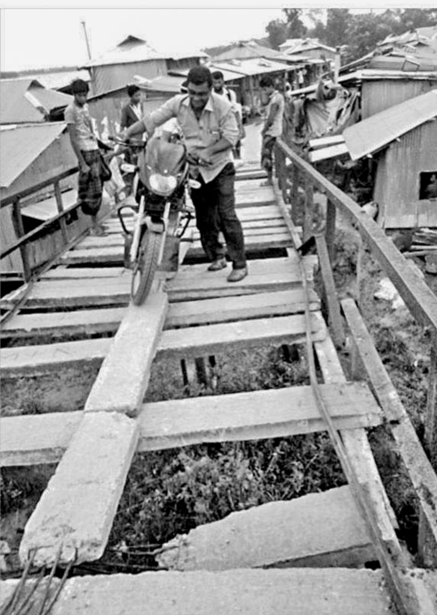
A man with a motorcycle crossing a dilapidated iron bridge on Kumirmara canal in Kalapara upazila of Patuakhali, risking his life. The photo was taken recently.
