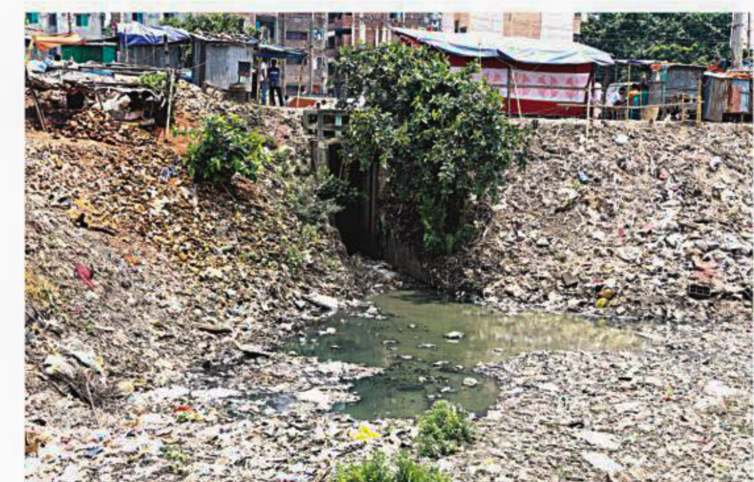
A sluice gate of the western flood protection embankment (Beribadh) in the capital's Nawabganj area. PHOTO: PRABIR DAS
