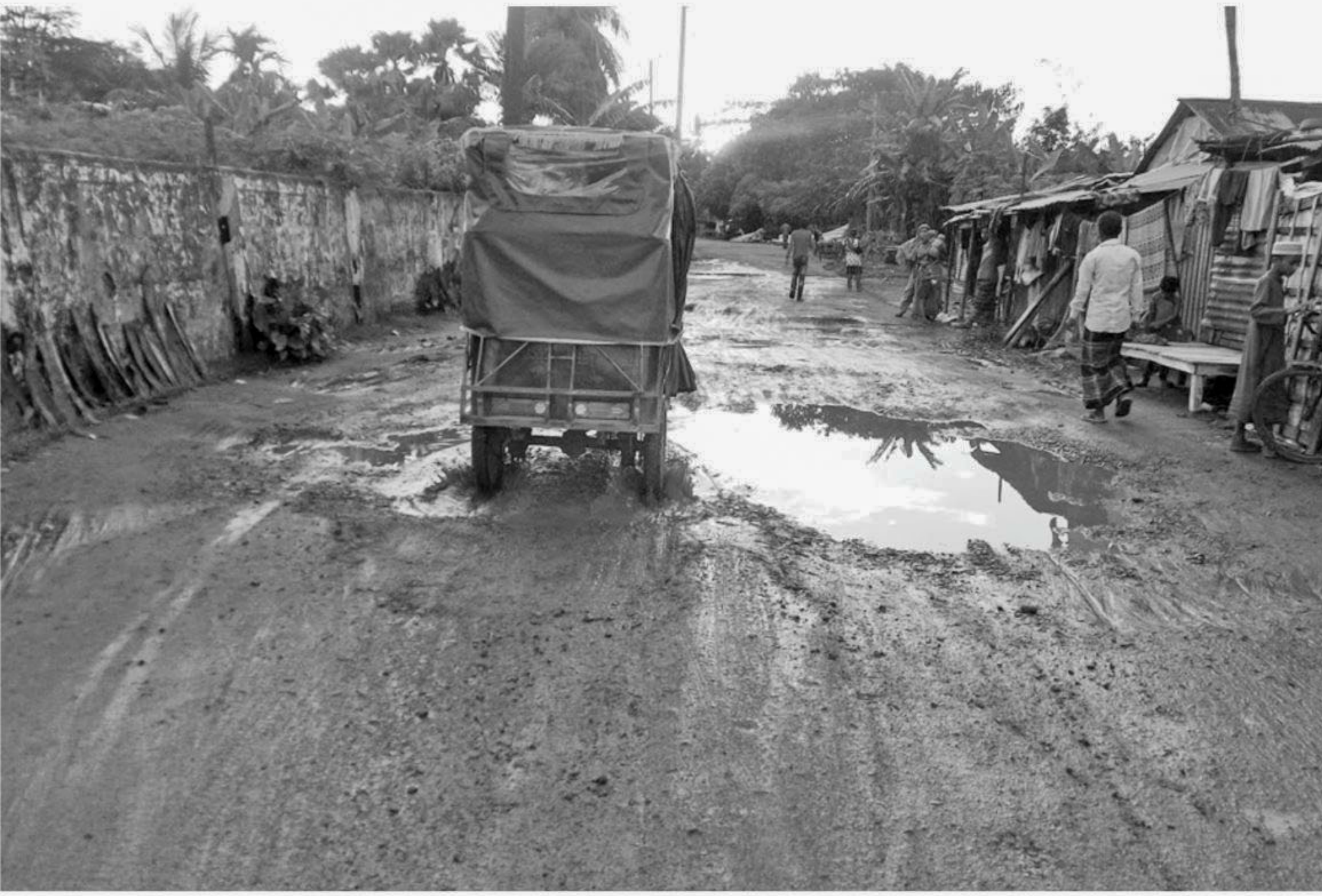
At least seven roads are lying dilapidated in Patuakhali town for long. The photo was taken at Toll Plaza road recently.
